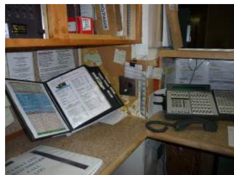
TELEPHONE SERVICES: Switchboard area in need of a remodel
