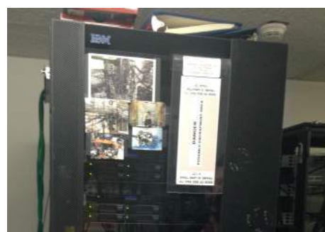
COMPUTER SERVICES: Secured server
