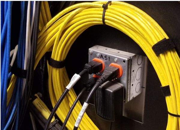
Existing Category 6a Cabling.
