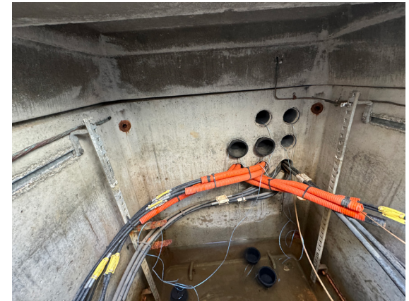
Existing Interbuilding Backbone Cabling.
