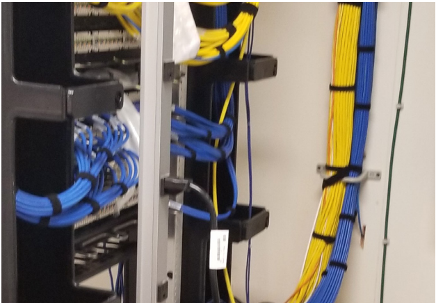
Existing Category 5e Cabling.
