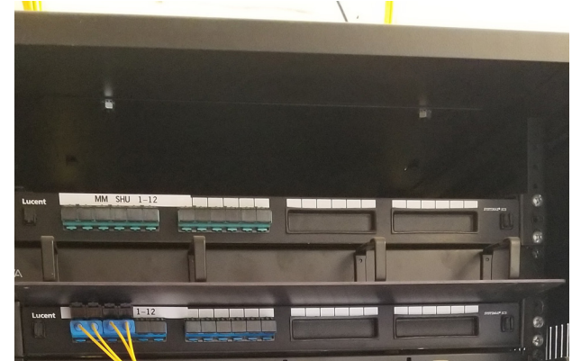
Existing Fiber Patching.
