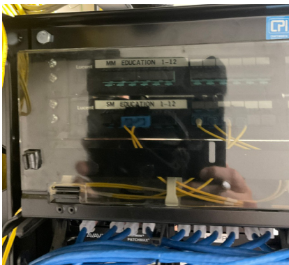
Existing Fiber Patching.
