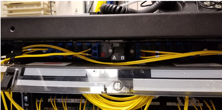
Existing Fiber Patching.
