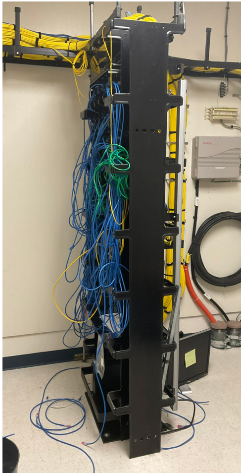
Existing Telecom Rack.
