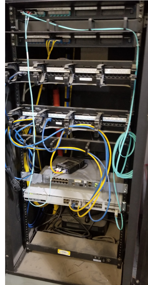
Existing Telecom Cabinet.
