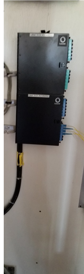
Existing Fiber Cabinet.
