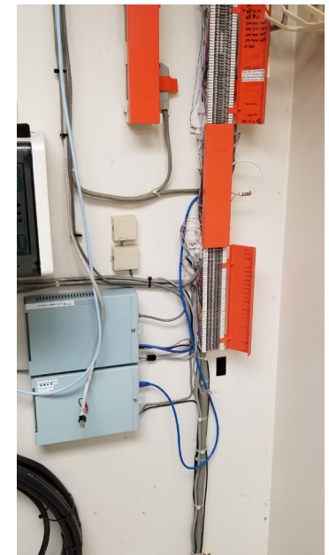
Existing Voice Patching.
