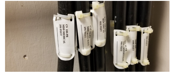
Existing Copper Backbone.
