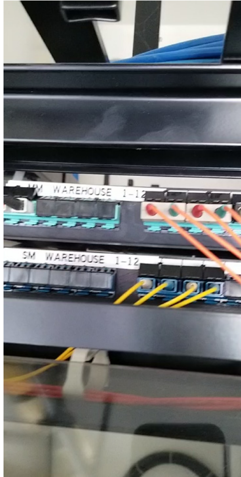
Existing Fiber Patching.
