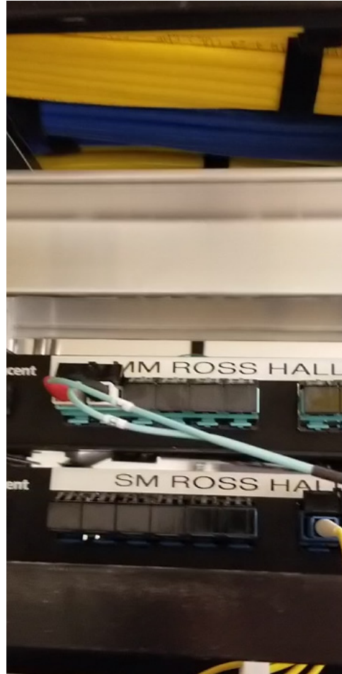
Existing Fiber Patching.
