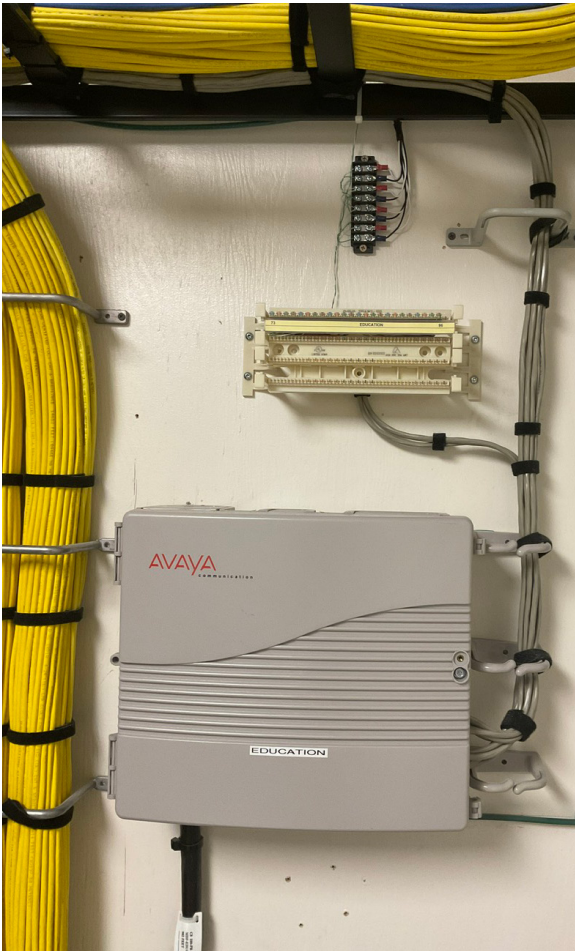
Existing Voice Patching.
