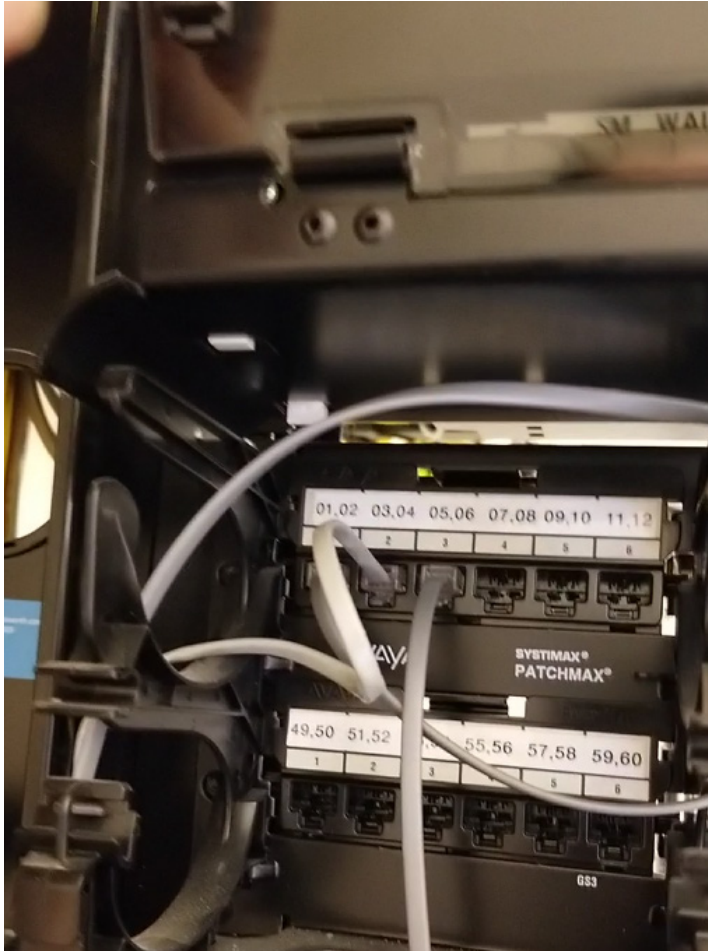
Existing Voice Patching.
