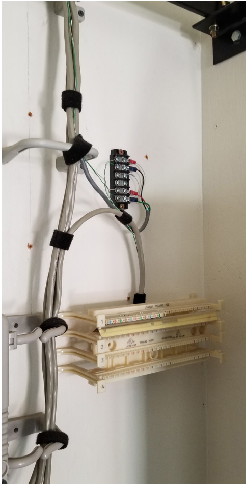
Existing Voice Patching.
