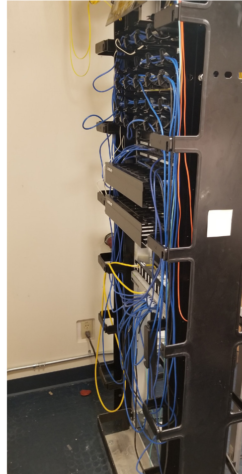
Existing Telecom Rack.
