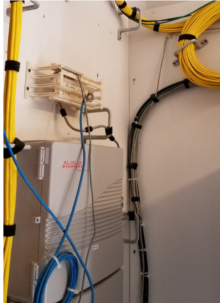
Existing Voice Patching.
