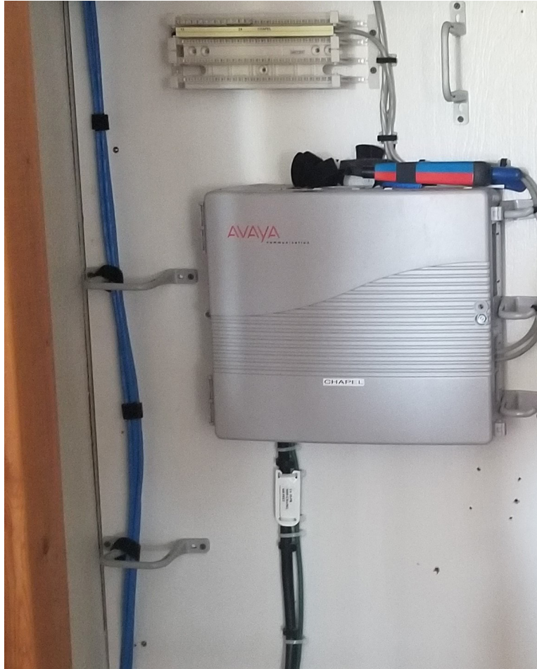
Existing Voice Patching.
