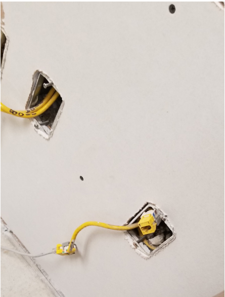
Existing Data Ports Without Cover Plates.
