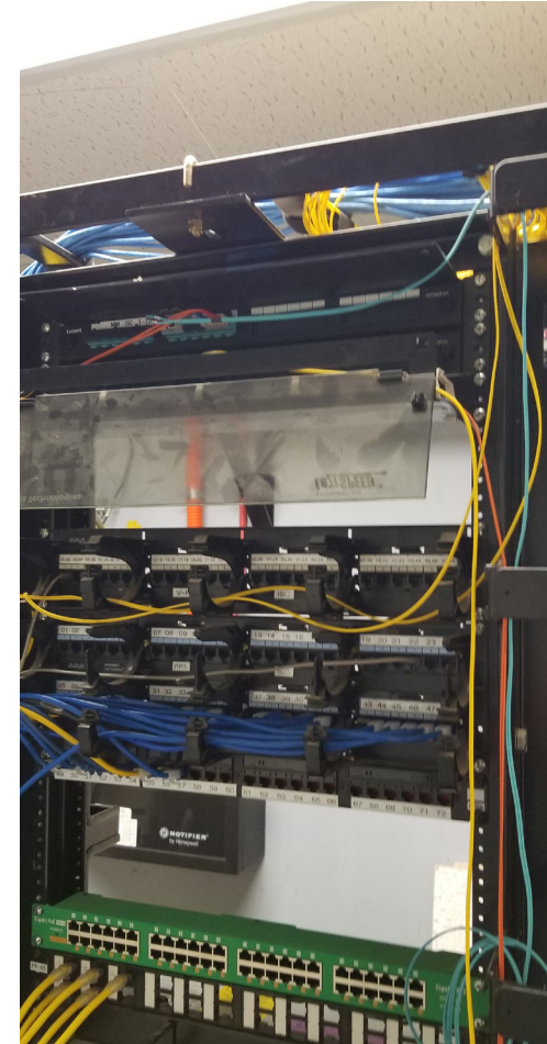
Existing Telecom Rack.
