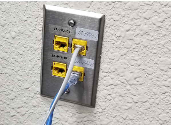
Existing Voice & Data Outlet.
