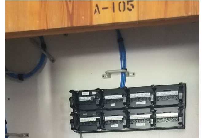
Existing Patch Panel.
