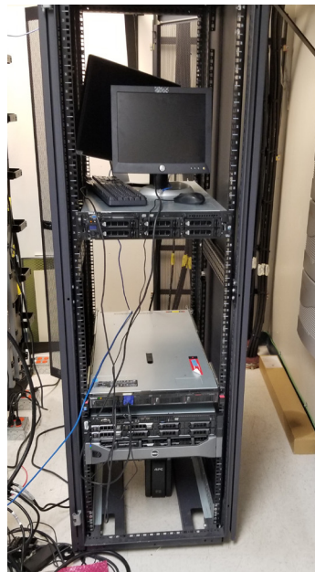
Existing Server Rack.
