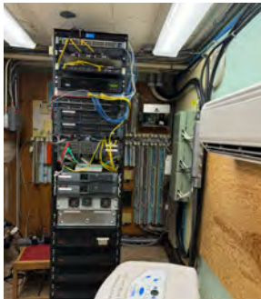
Existing Telecom Rack.
