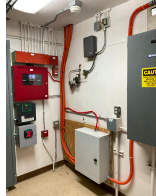
Existing Cross-Connect Room.
