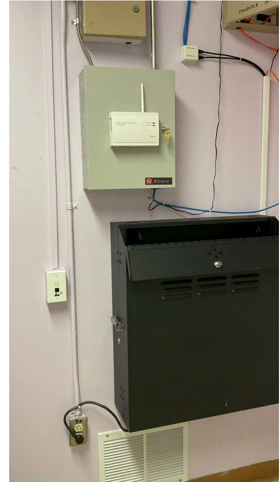
Existing Telecom Cabinet.
