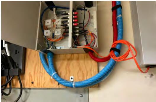
Existing Fiber Patching.
