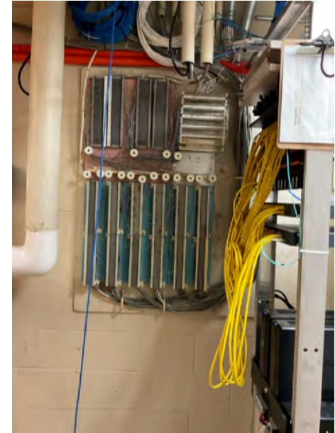
Existing Voice Patching.
