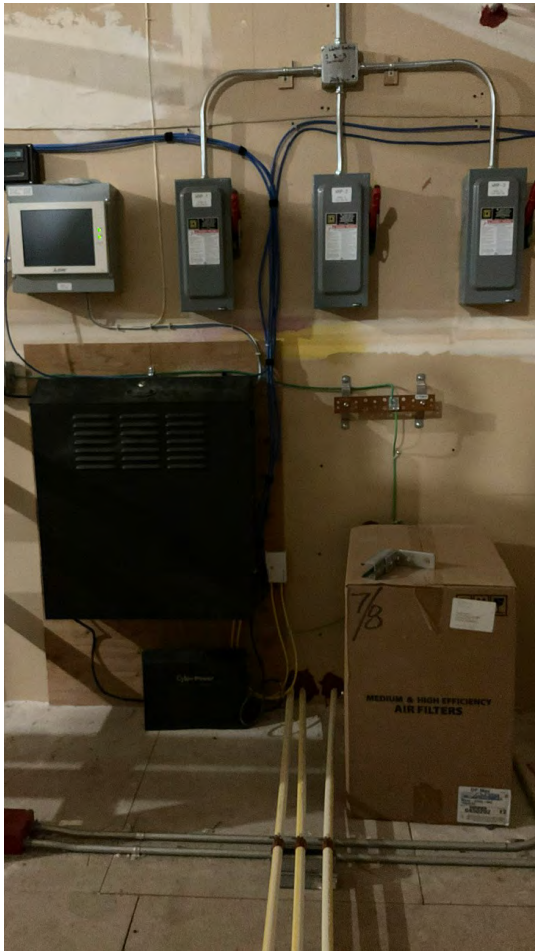
Existing Telecom Cabinet.
