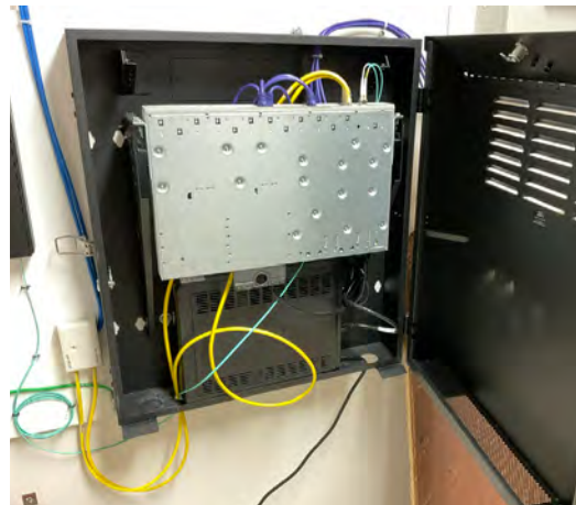
Existing Telecom Cabinet.
