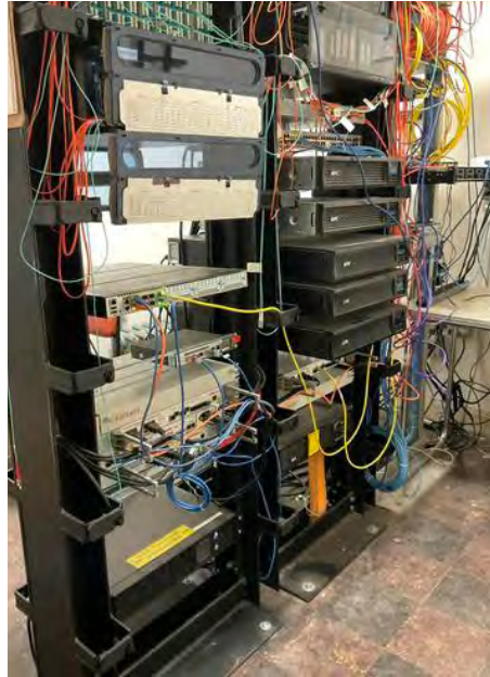
Existing Telecom Racks.
