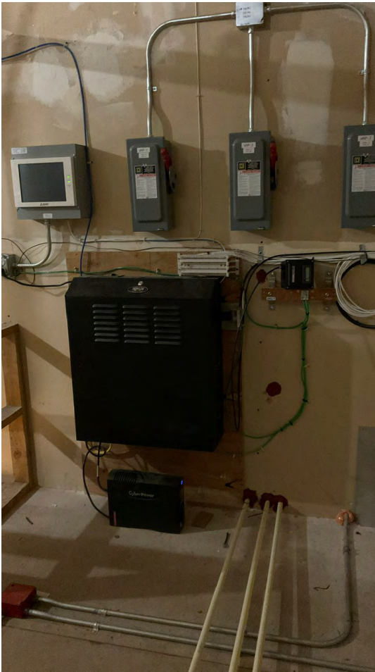
Existing Telecom Cabinet.
