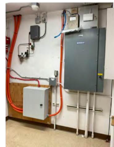
Existing Cross-Connect Room.
