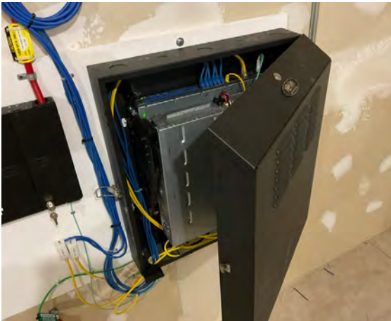
Existing Telecom Cabinet.
