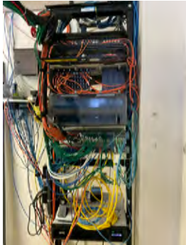
Existing Telecom Rack.
