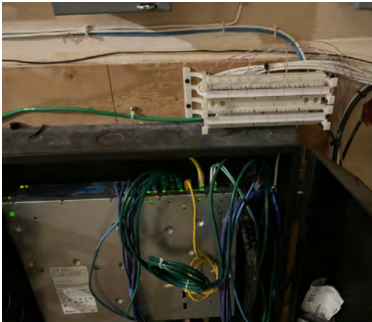
Existing Voice Patching.
