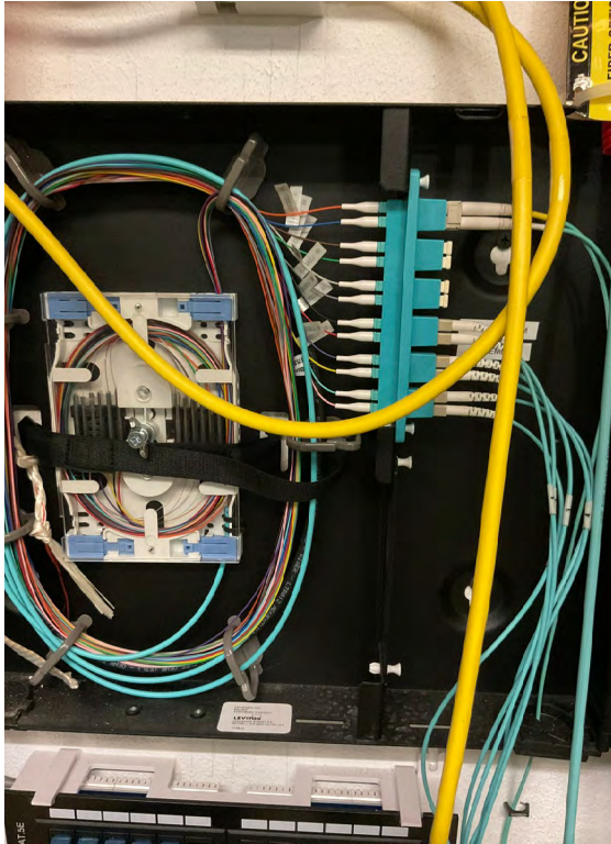
Existing Fiber Patching.
