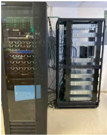
Existing UPS & Server Racks.
