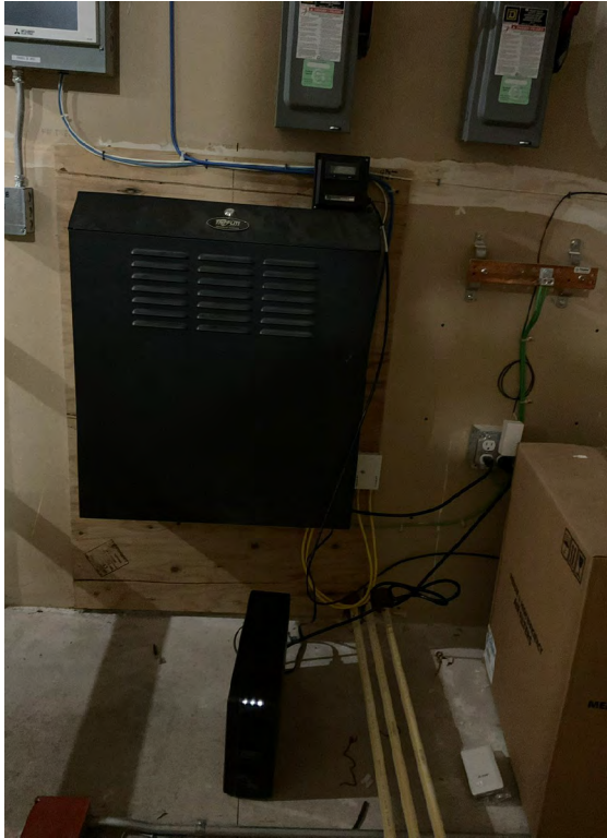
Existing Telecom Cabinet.
