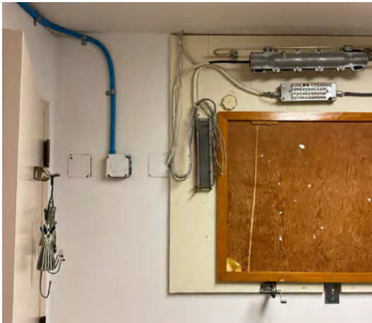
Existing Voice Patching.
