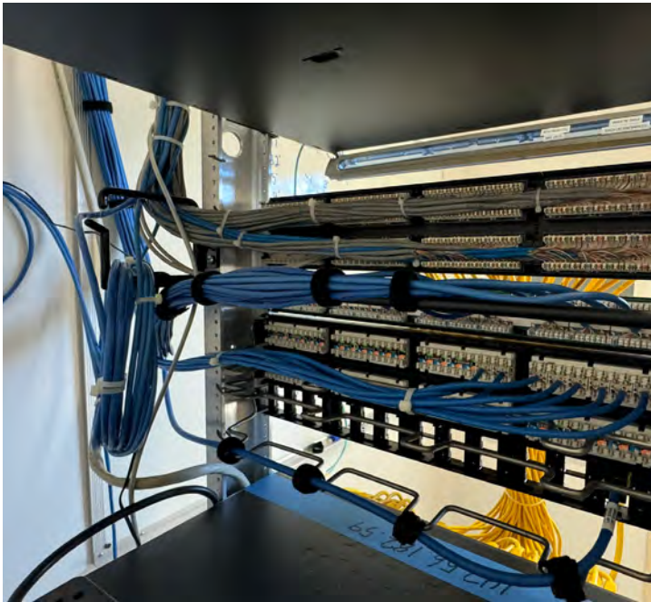
Existing Horizontal Cabling Patching.
