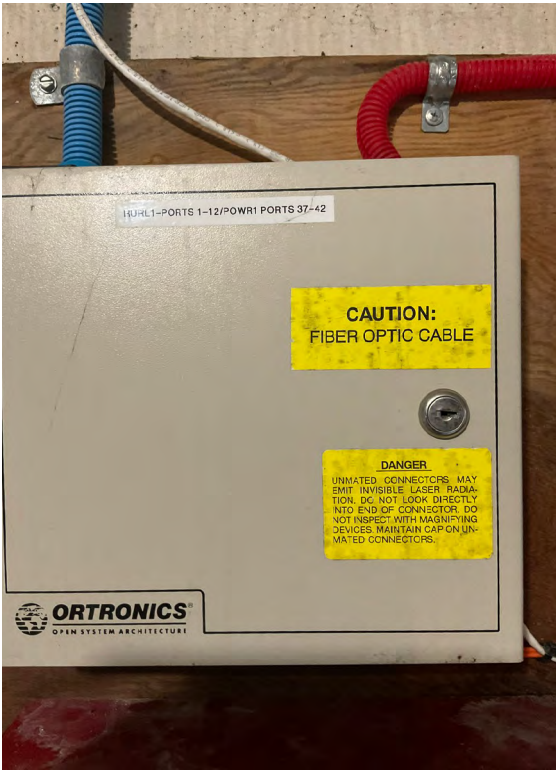
Existing Fiber Cabinet.
