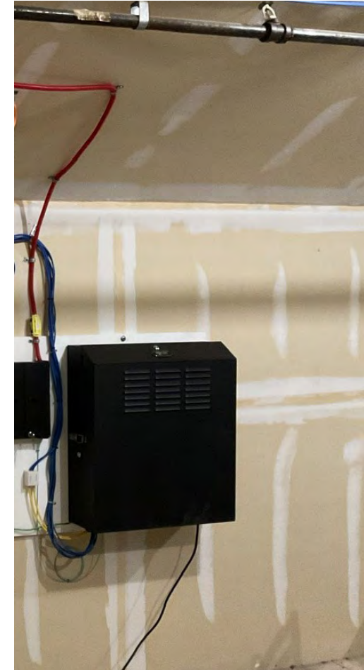
Existing Telecom Cabinet.
