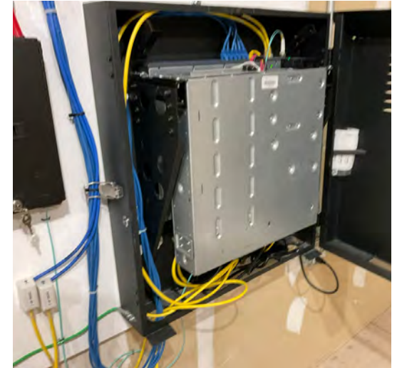
Existing Fiber Patching.
