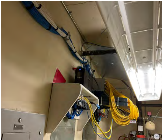
Existing Telecom Equipment.
