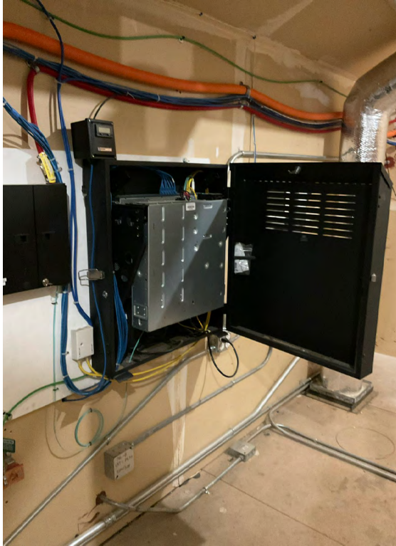
Existing Telecom Cabinet.
