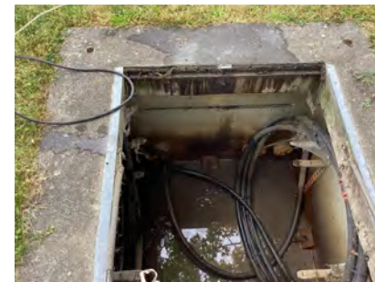
Existing Interbuilding Backbone Cabling.
