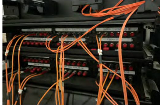
Existing Fiber Patching.
