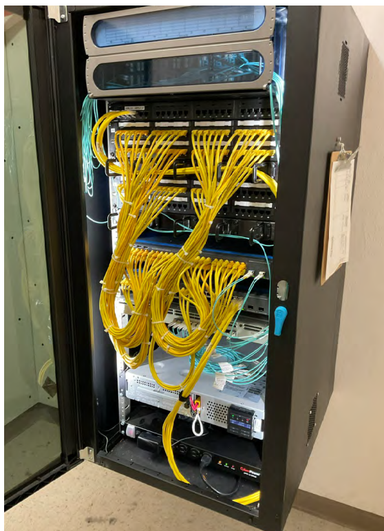
Existing Telecom Cabinet.
