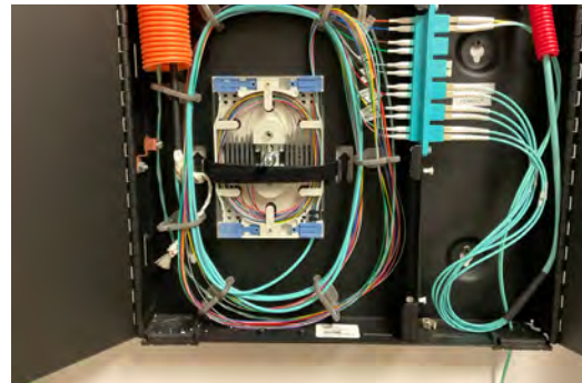
Existing Fiber Patching.
