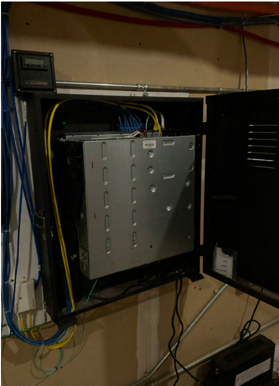
Existing Telecom Cabinet.
