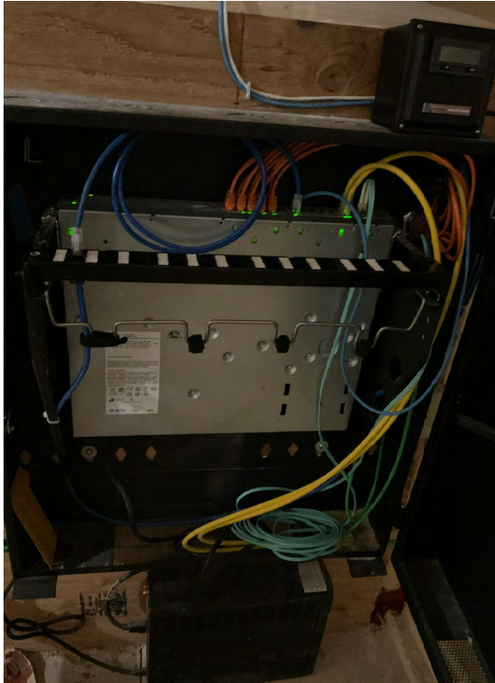
Existing Telecom Cabinet.
