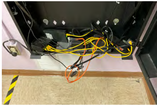
Existing Fiber & Data Patching.
