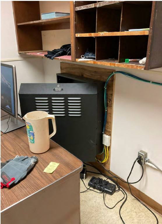
Existing Telecom Cabinet.
