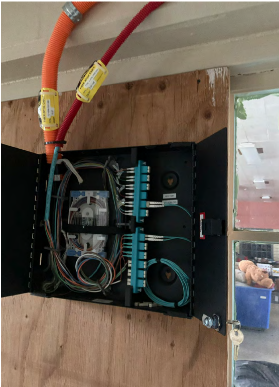
Existing Fiber Cabinet.
