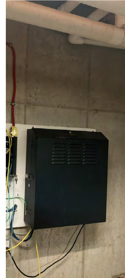
Existing Telecom Cabinet.
