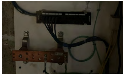
Existing Category 5e Patch Panel.
