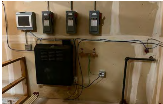
Existing Telecom Cabinet.
