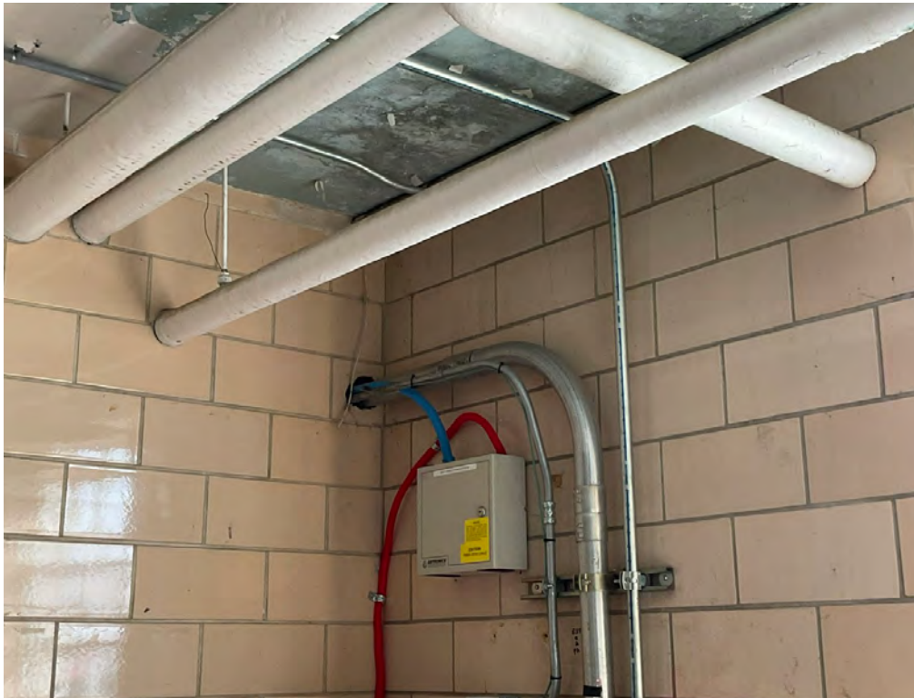
Existing Fiber Cabinet.
