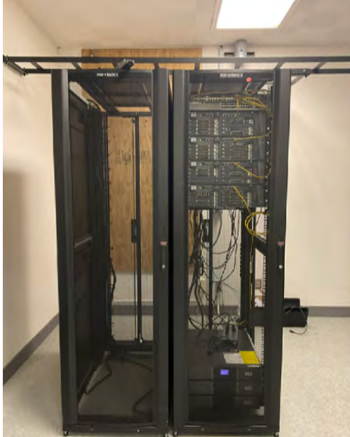
Existing Telecom Racks.
