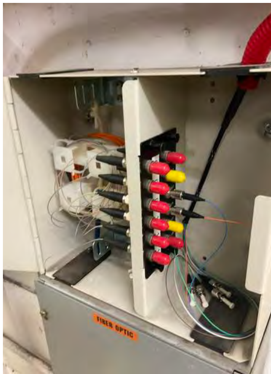
Existing Fiber Patching.
