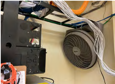
Existing Fan Used for Cooling.
