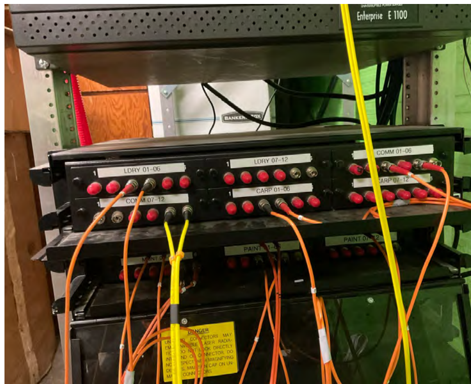
Existing Fiber Patching.
