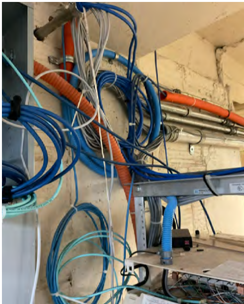
Existing Cables in Telecom Room.
