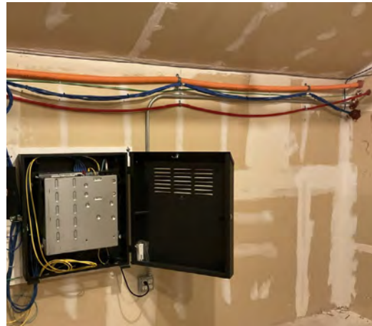
Existing Telecom Cabinet.
