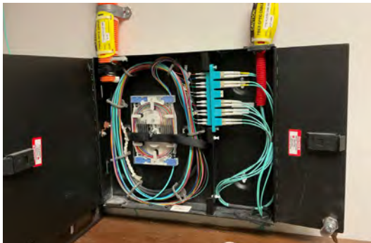
Existing Fiber Patching.
