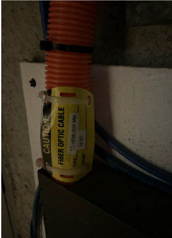
Existing SM Fiber Infrastructure.
