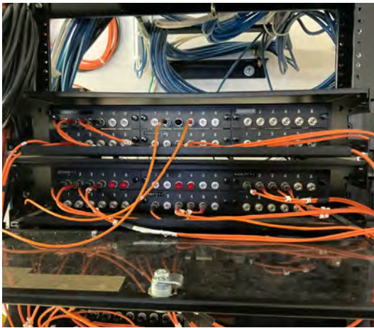
Existing Fiber Patching.
