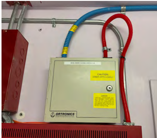
Existing Fiber Cabinet.
