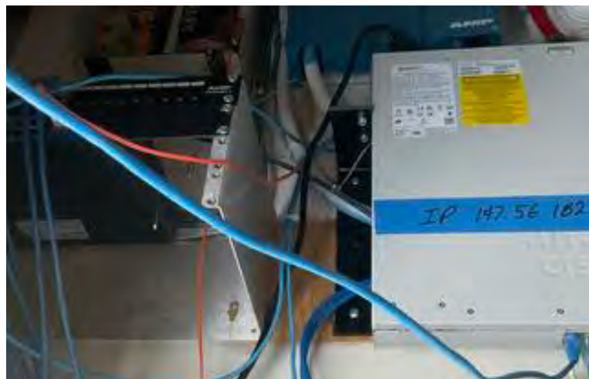
Existing Telecom Room.
