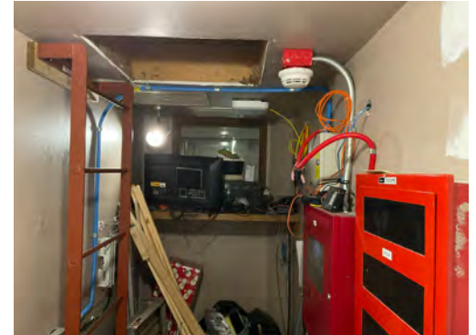
Existing Telecom Room.
