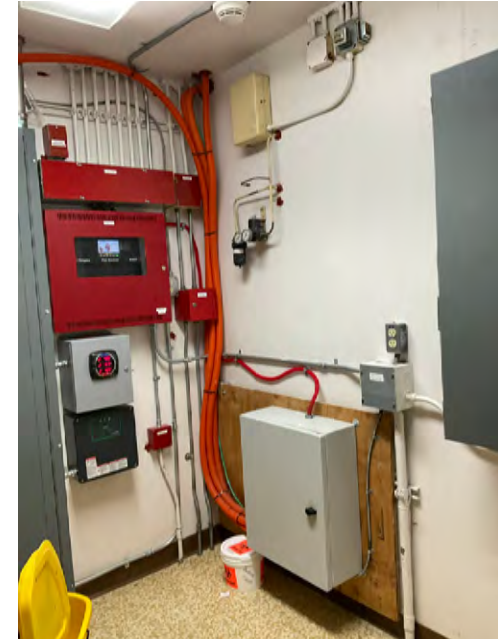
Existing Cross-Connect Room.
