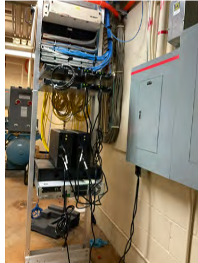
Existing Telecom Rack.
