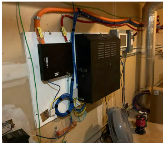
Existing Telecom Cabinet.
