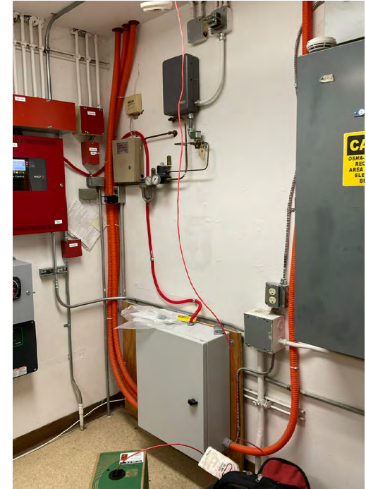
Existing Cross-Connect Room.
