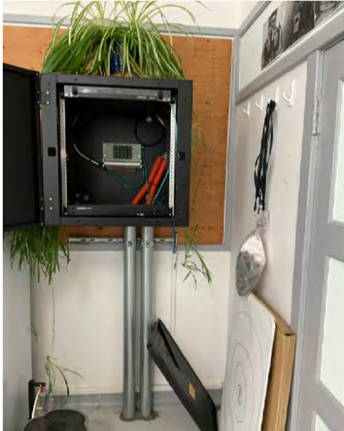
Existing Telecom Cabinet.
