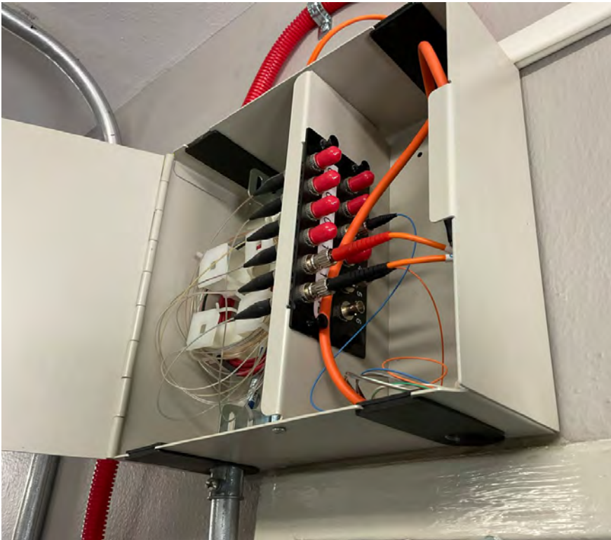
Existing Fiber Patching.
