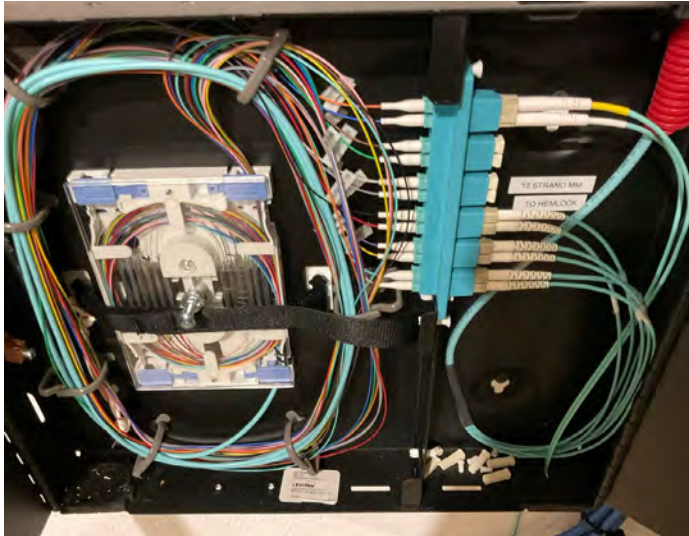
Existing Fiber Patching.
