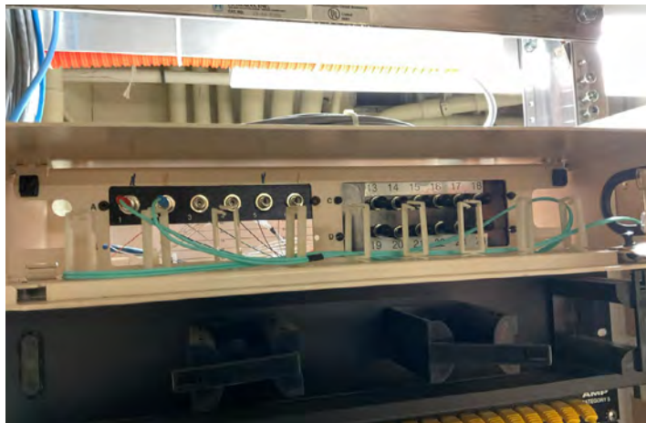
Existing Voice Patching.
