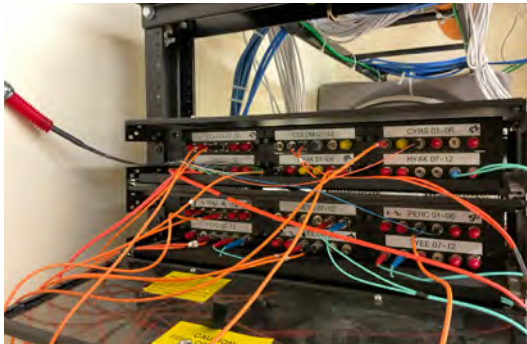
Existing Fiber Patching.
