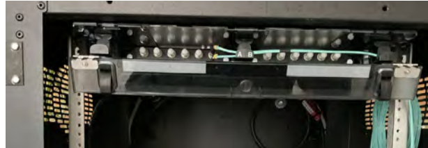
Existing Fiber Patching.
