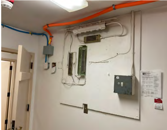
Existing Voice Patching.
