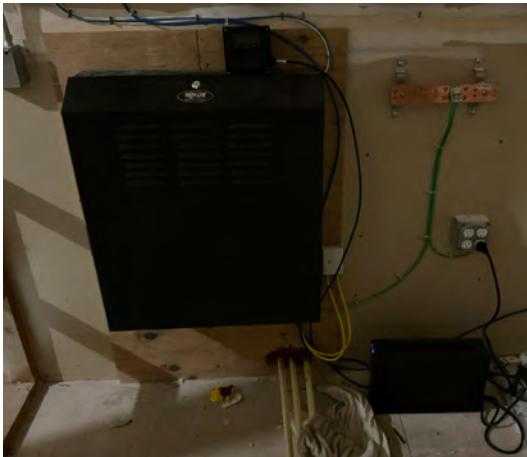
Existing Telecom Cabinet.
