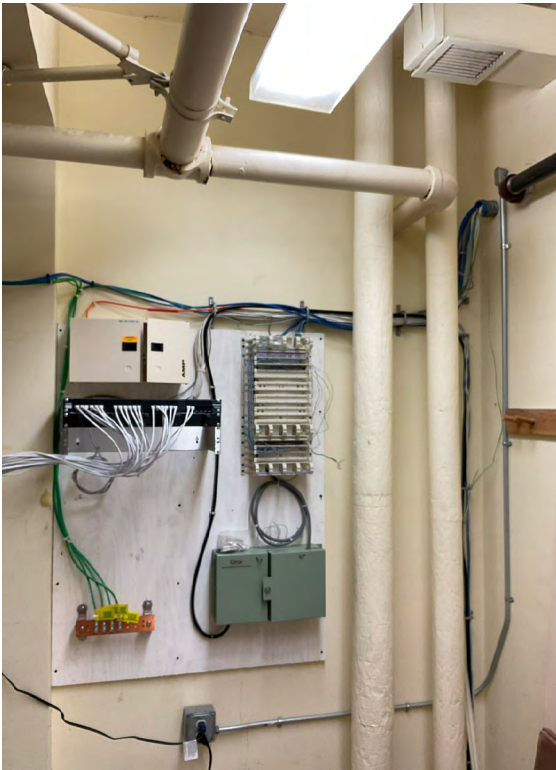
Existing Voice & Data Patching.
