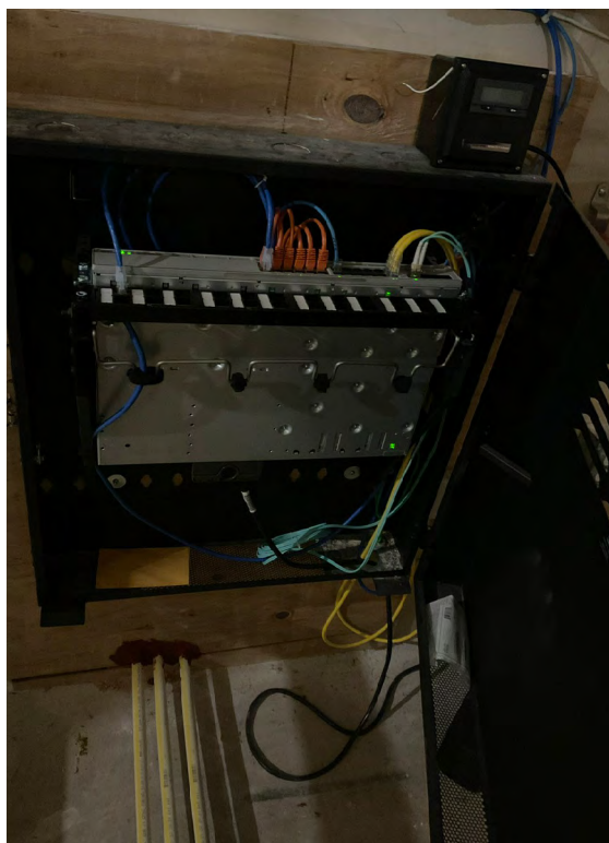
Existing Telecom Cabinet.
