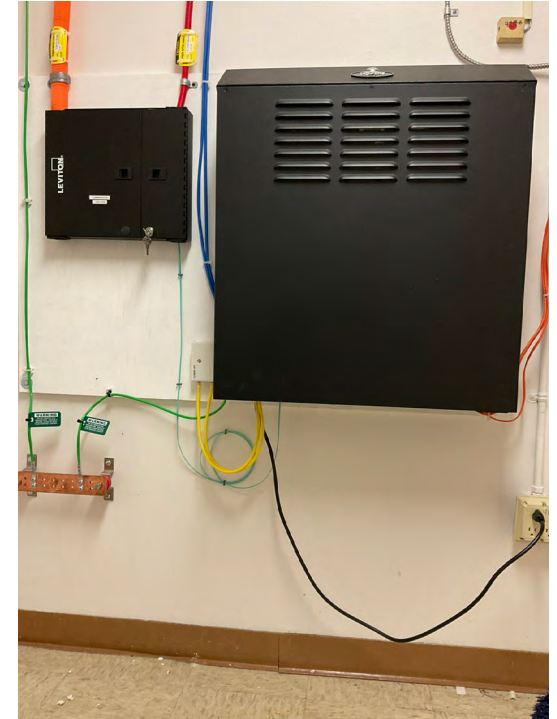
Existing Telecom Cabinet.
