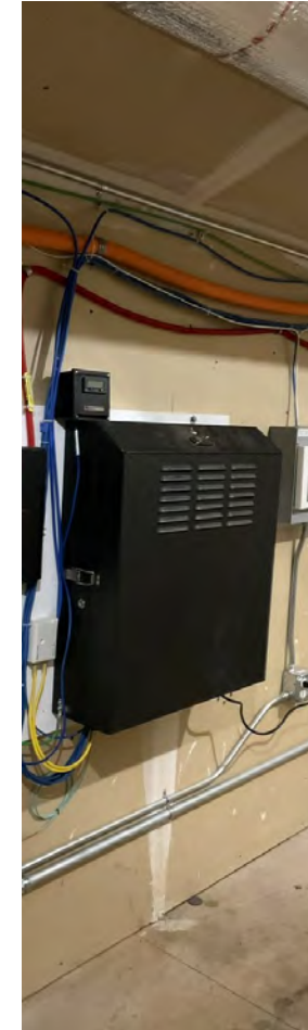
Existing Telecom Cabinet.
