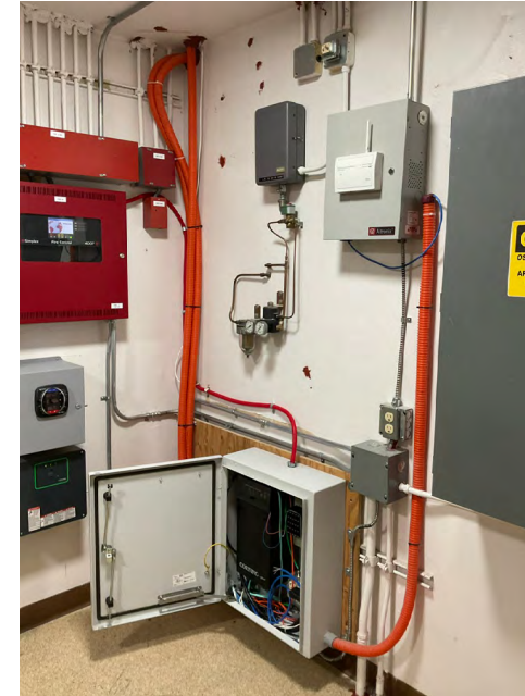
Existing Cross-Connect Room.
