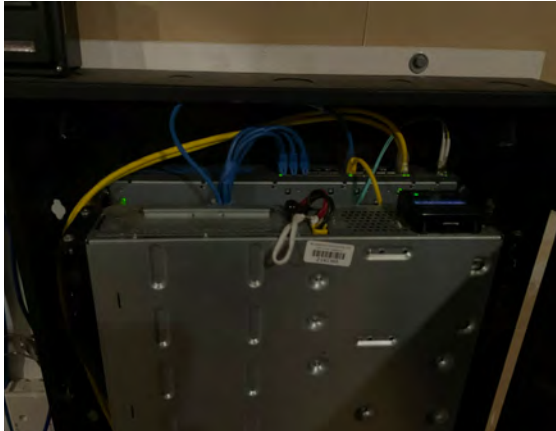
Existing Fiber & Data Patching.
