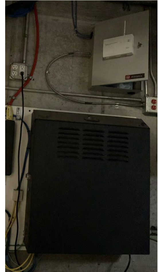
Existing Telecom Cabinet.
