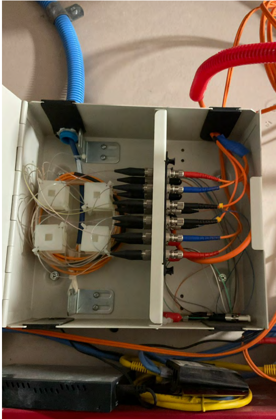
Existing Fiber Patching.
