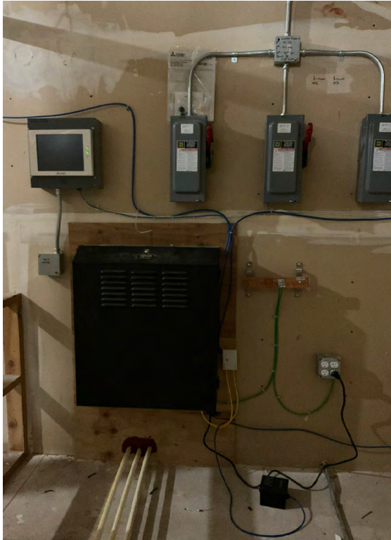
Existing Telecom Cabinet.
