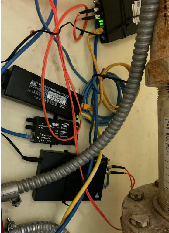
Existing Fiber Patching.
