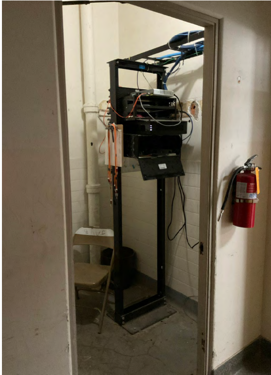
Existing Telecom Rack.
