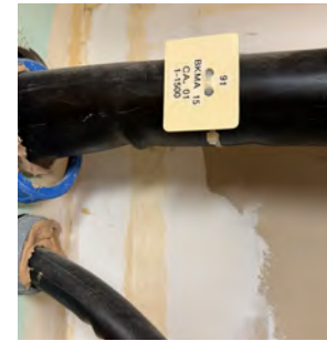
Existing Copper Backbone.
