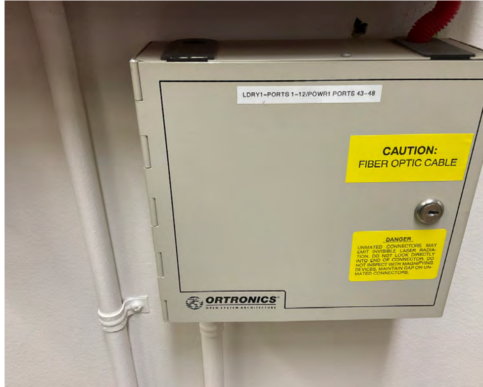
Existing Fiber Cabinet.
