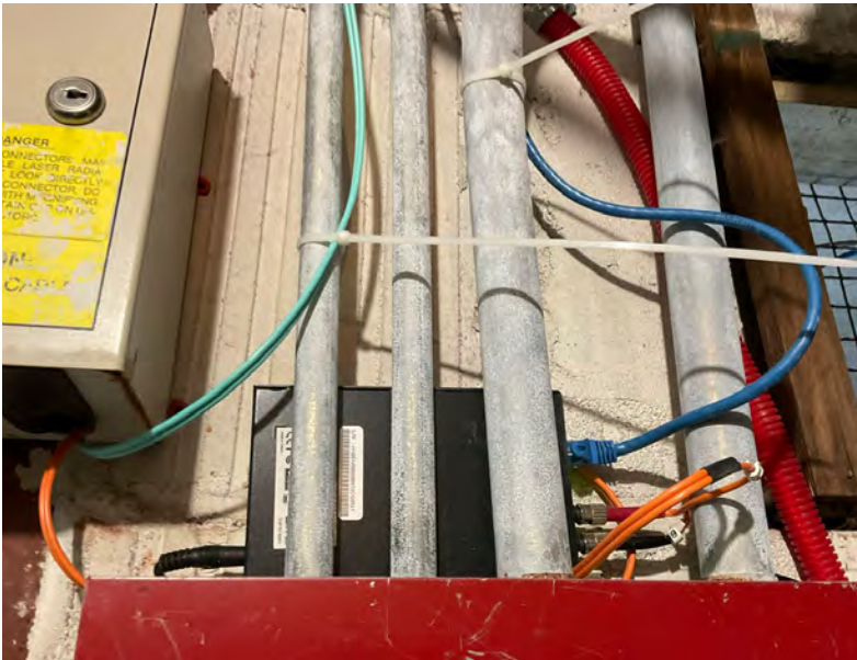
Existing Fiber & Data Patching.
