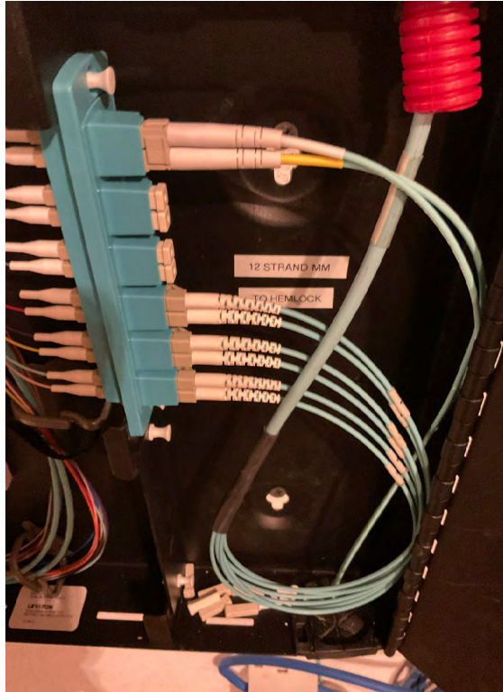
Existing Fiber Patching.
