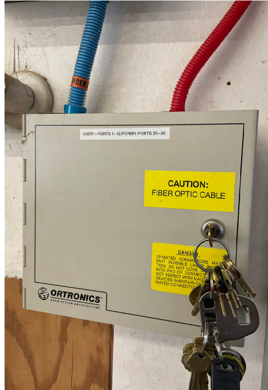
Existing Fiber Cabinet.
