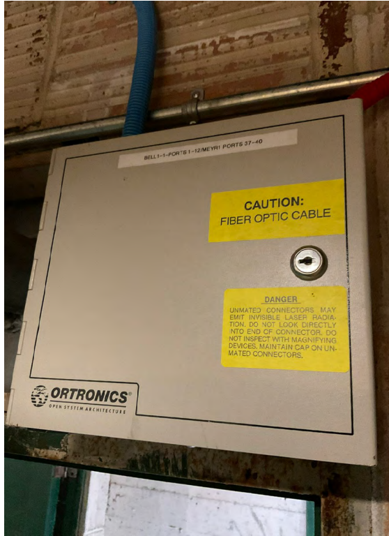
Existing Fiber Cabinet.
