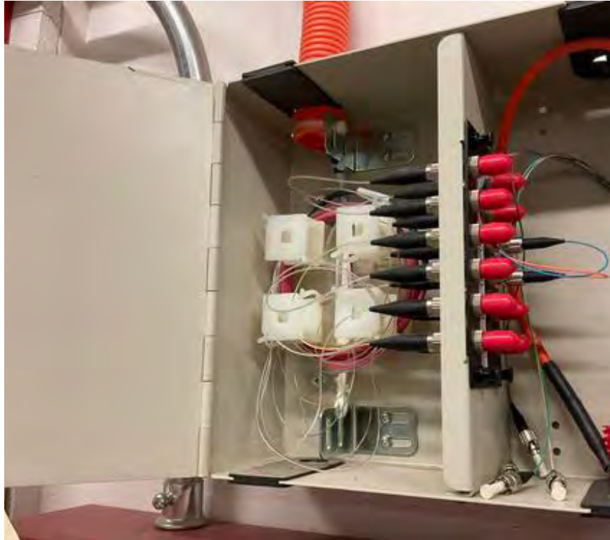
Existing Fiber Patching.
