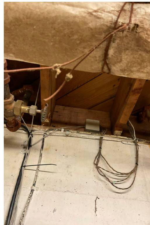
Existing Category 3 Cabling.
