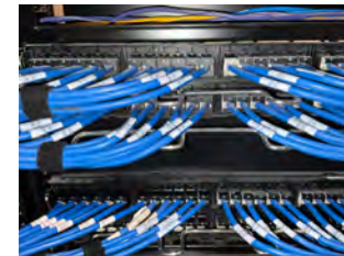
Existing Category 6A Cabling.
