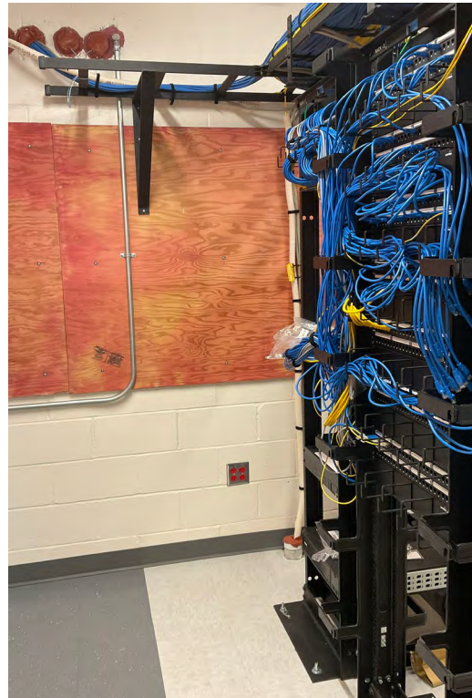
Existing Telecom Racks.
