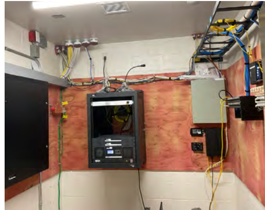
Existing Telecom Room.
