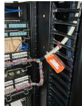
Existing Voice Patching (2).
