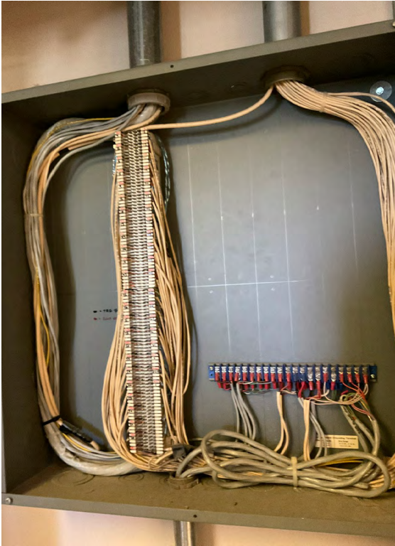
Existing Voice Patching.
