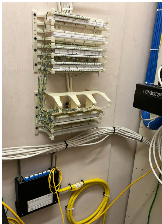
Existing Fiber and Voice Patching.
