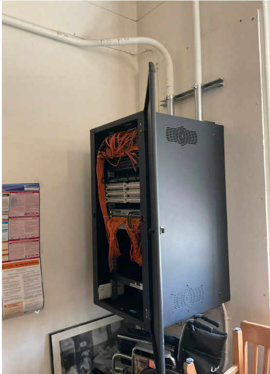
Existing Telecom Enclosure.
