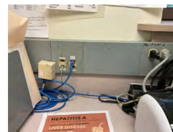
Existing Telecom Outlets.
