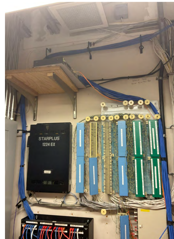
Existing Voice Patching.
