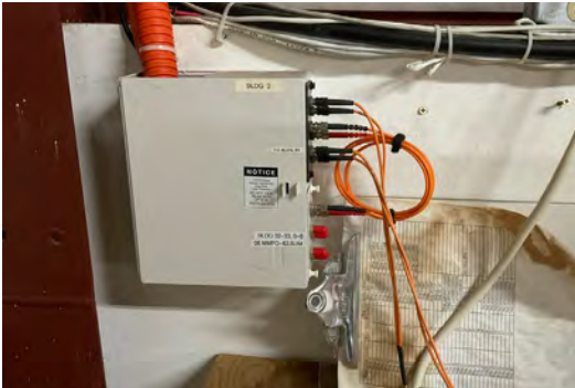
Existing Fiber Cabinet.
