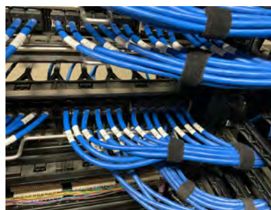
Existing Category 6A Cabling.
