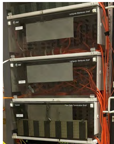
Existing Fiber Patching.
