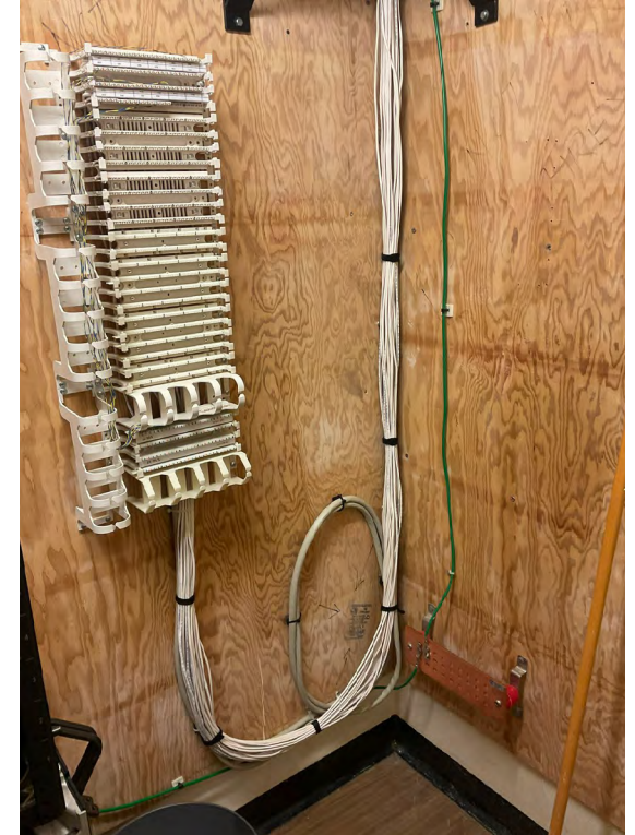
Existing Voice Patching.
