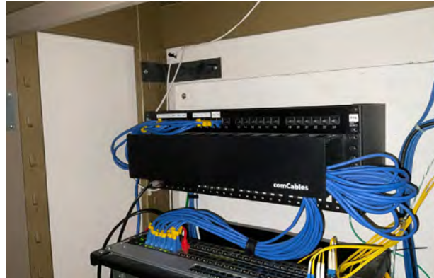
Existing Voice and Data Patching.
