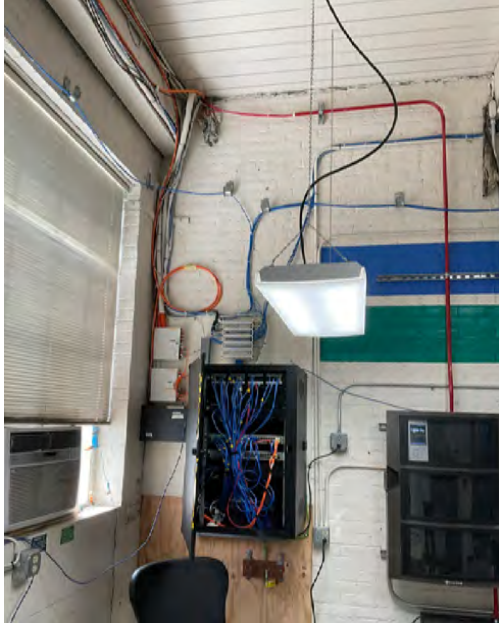
Existing Telecom Enclosure.
