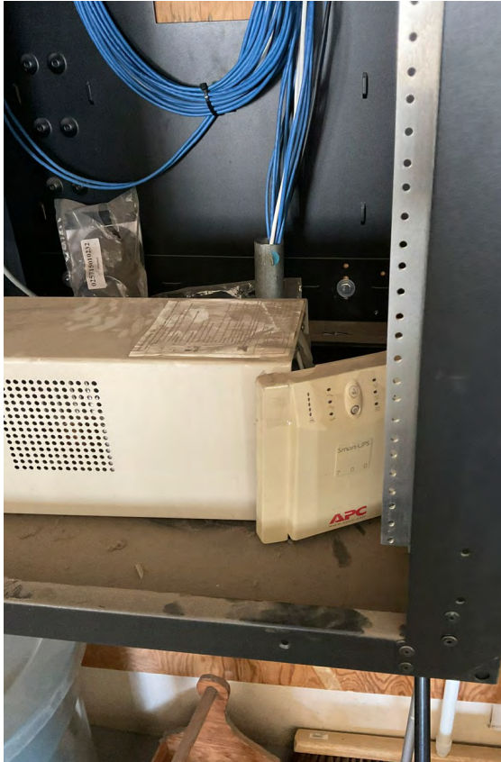
Existing Broken UPS.
