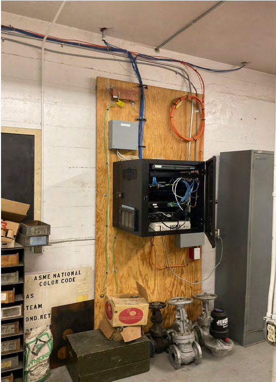
Existing Telecom Enclosure.
