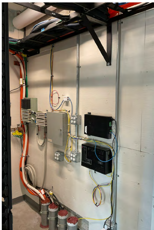
Existing Wall-Mounted Equipment.
