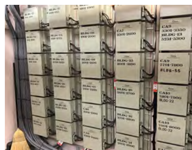
Existing Category 3 Backbone Cabling.
