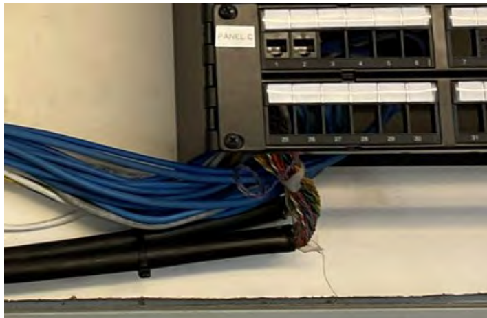
Existing Horizontal Cabling.
