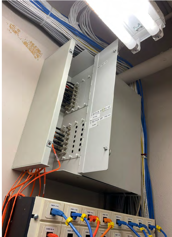
Existing Fiber Cabinet.
