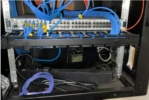
Existing Telecom Cabinet.
