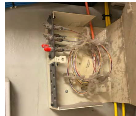
Existing Unused Fiber.
