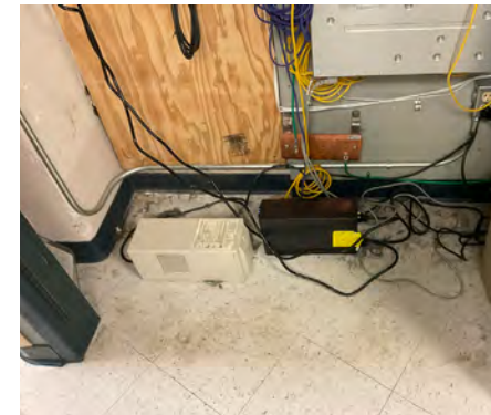
Existing Grounding and UPS.
