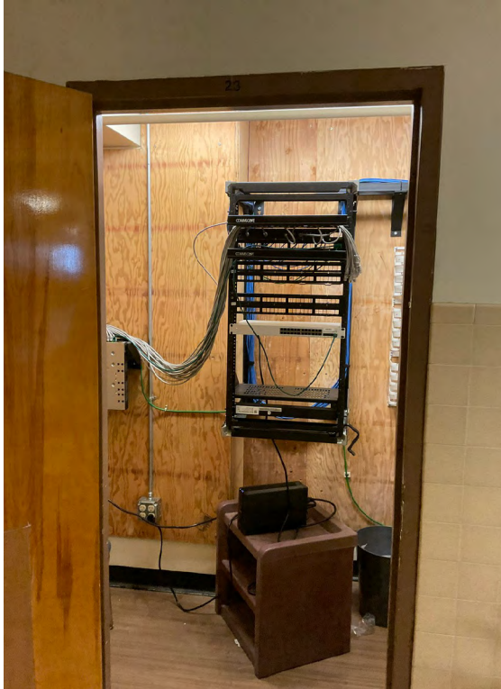
Existing Telecom Rack.
