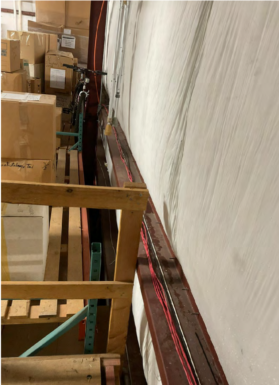
Existing Cable Routing.
