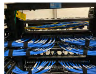
Existing Category 6A Patching.
