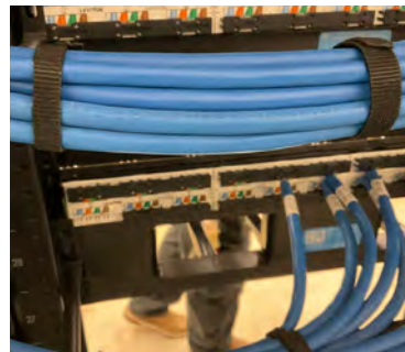
Existing Category 6A Cabling.
