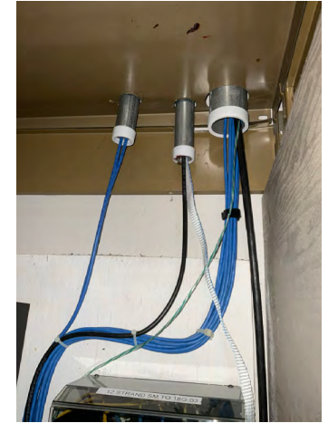
Existing Horizontal Cabling.
