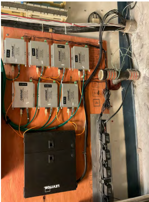
Existing Media Converters.
