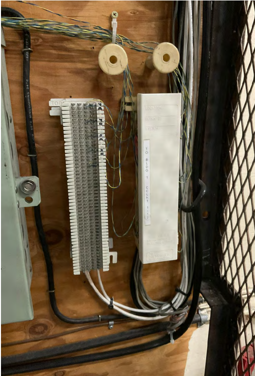
Existing Voice Patching.
