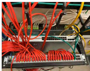
Existing Telecom Rack.
