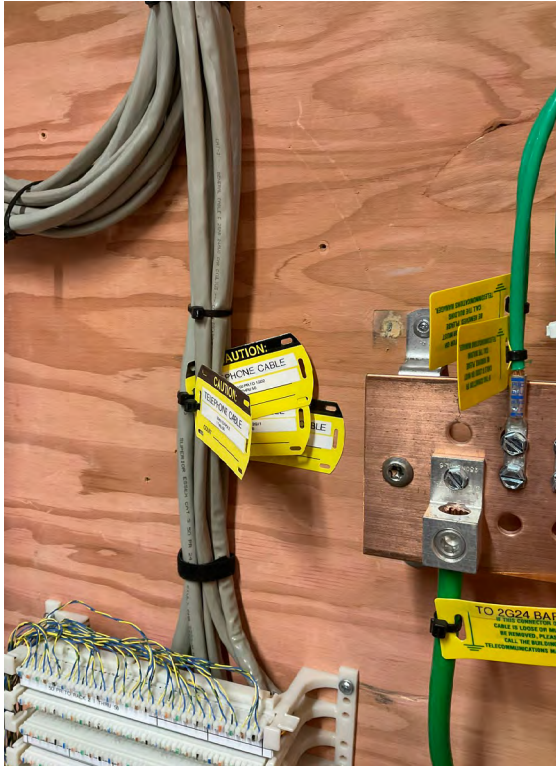
Existing Voice Patching.
