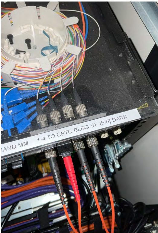
Existing Fiber Cabinet.
