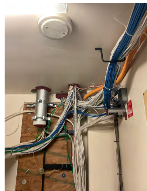
Existing Horizontal Cabling (2)
