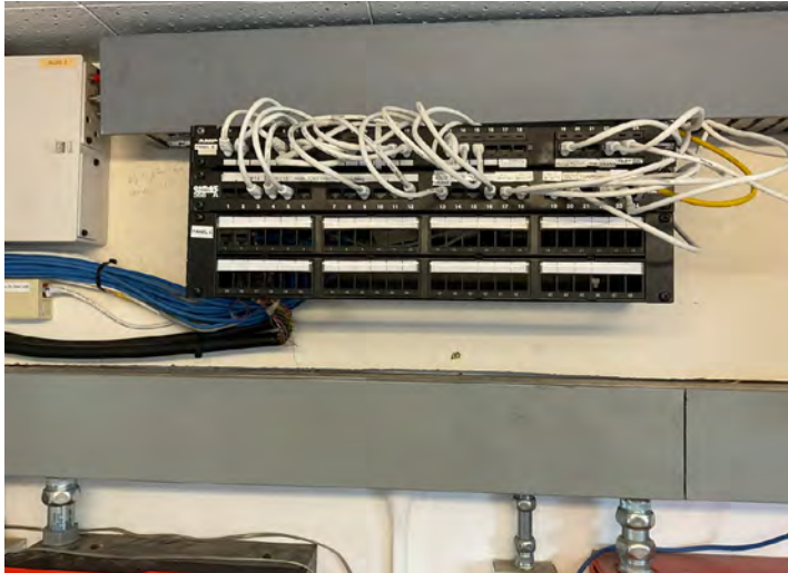
Existing Data & Voice Patching.
