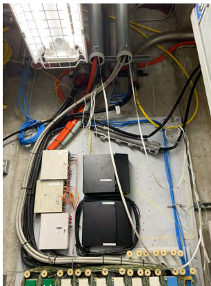
Existing Fiber Cabinets.
