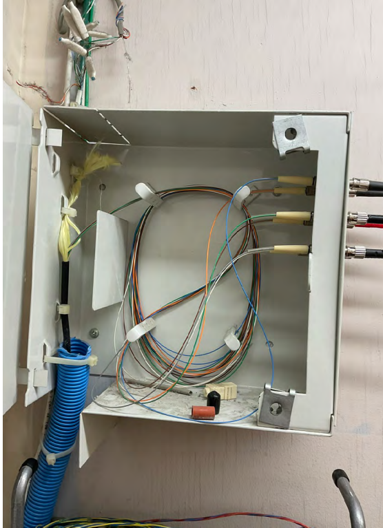
Existing Fiber Patching.
