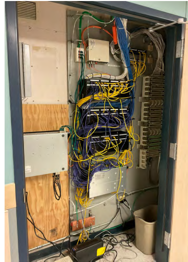
Existing Telecom Room.
