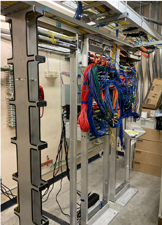
Existing Telecom Rack.
