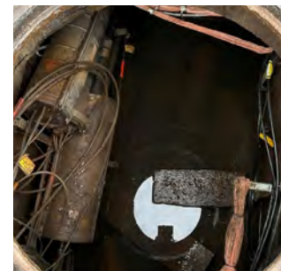
Existing Fiber and Copper Splices.
