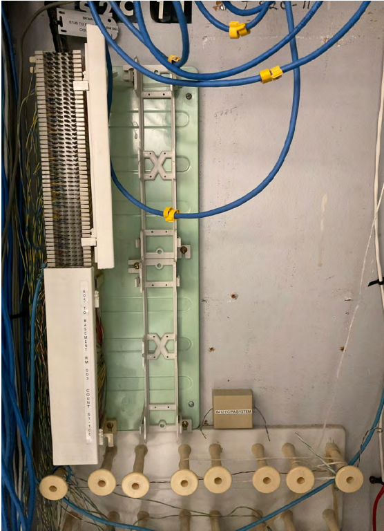
Existing Voice Patching.
