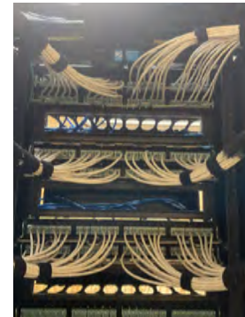
Existing Category 5e Cabling.
