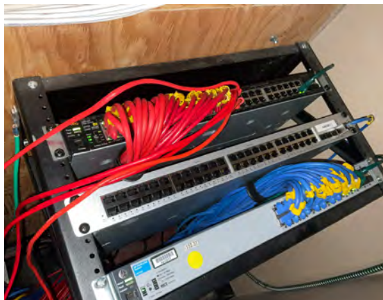
Existing Telecom Rack.
