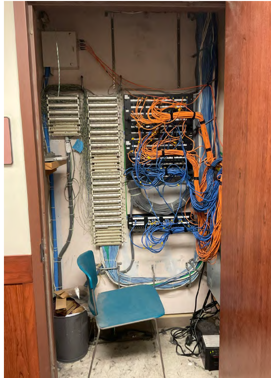
Existing Telecom Room.
