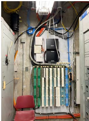
Existing Telecom Room.
