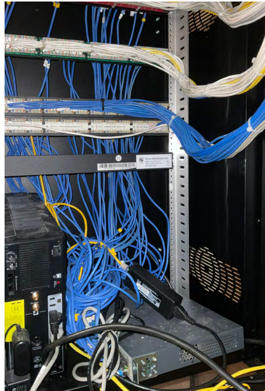
Existing Voice and Data Patching.
