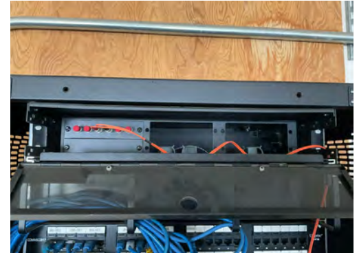
Existing Fiber Patching.
