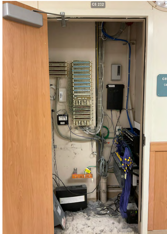
Existing Telecom Room.
