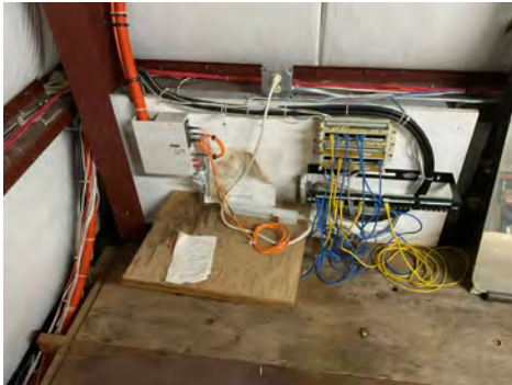
Existing Telecom Equipment.
