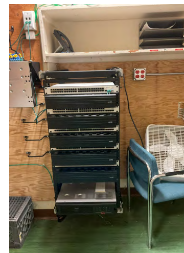
Existing Telecom Rack.
