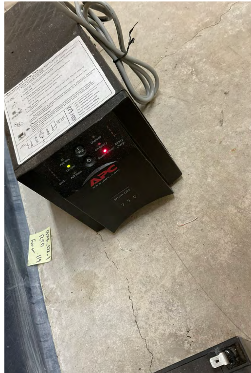
Existing Failing UPS.
