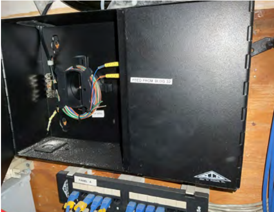
Existing Cut Fiber.
