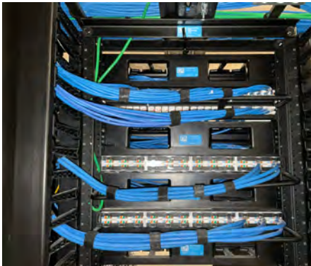
Existing Category 6A Cabling.
