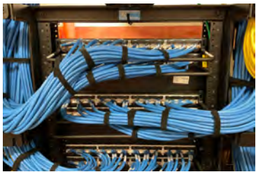
Existing Category 6A Cabling.
