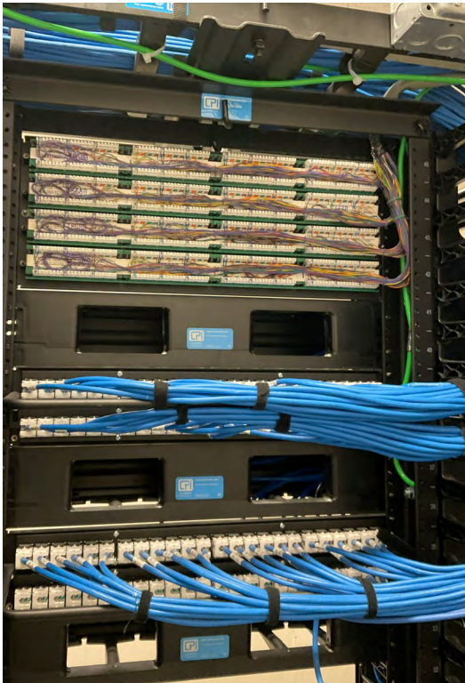
Existing Voice Patching.
