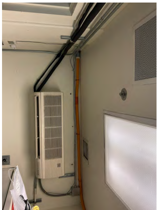
Existing Cooling Unit.
