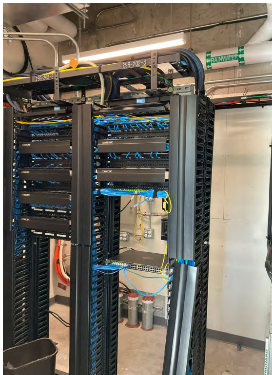
Existing Telecom Racks.
