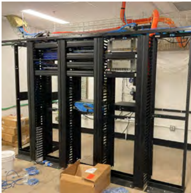
Existing Telecom Racks.
