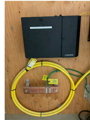
Existing Grounding and OFC.
