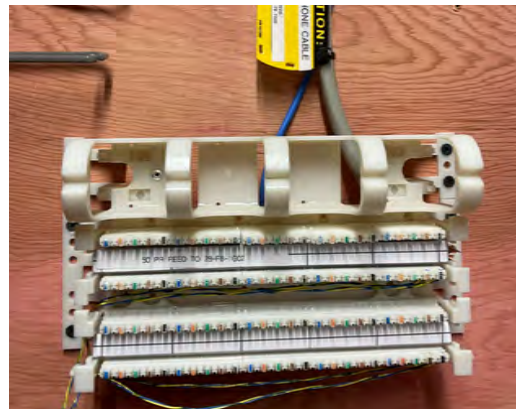
Existing Voice Patching.
