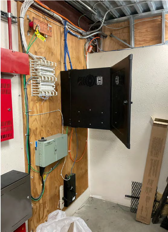
Existing Telecom Equipment.
