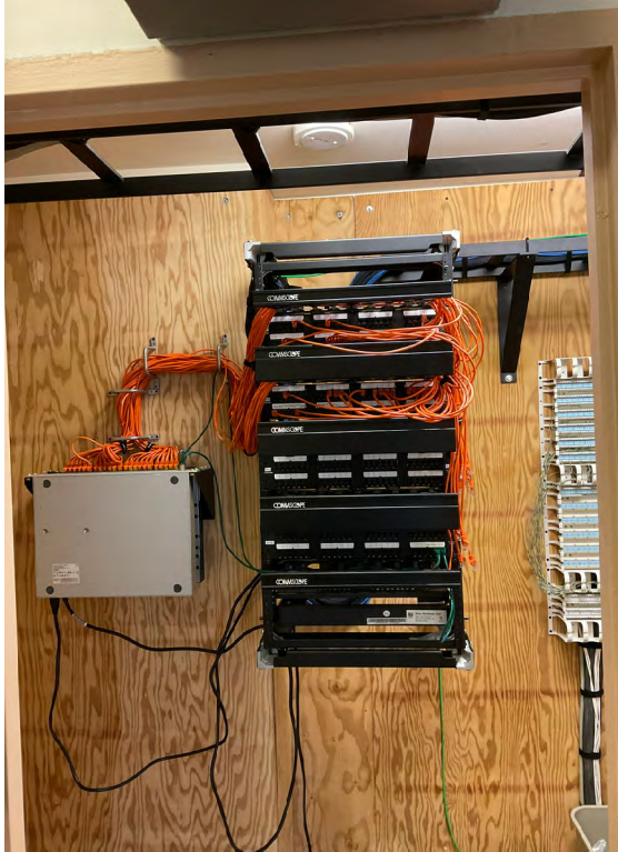
Existing Telecom Rack.
