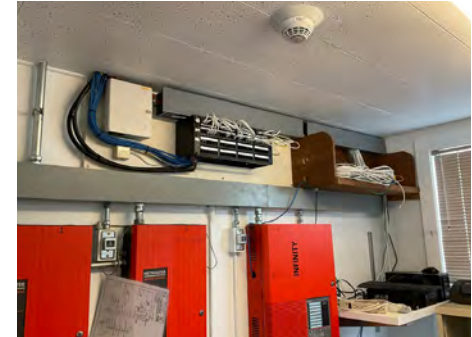
Existing Telecom Equipment.
