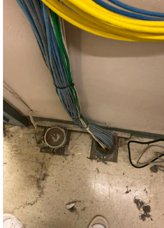
Existing Horizontal Cabling.
