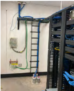
Existing Telecom Room.
