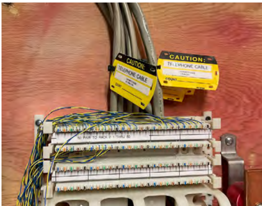
Existing Voice Patching.
