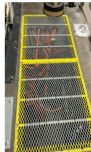
Existing Backbone Cabling In Bldg 18 Tunnel.
