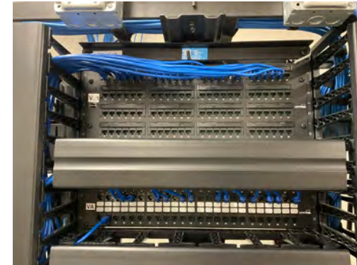
Existing Category 5e Patch Panels.
