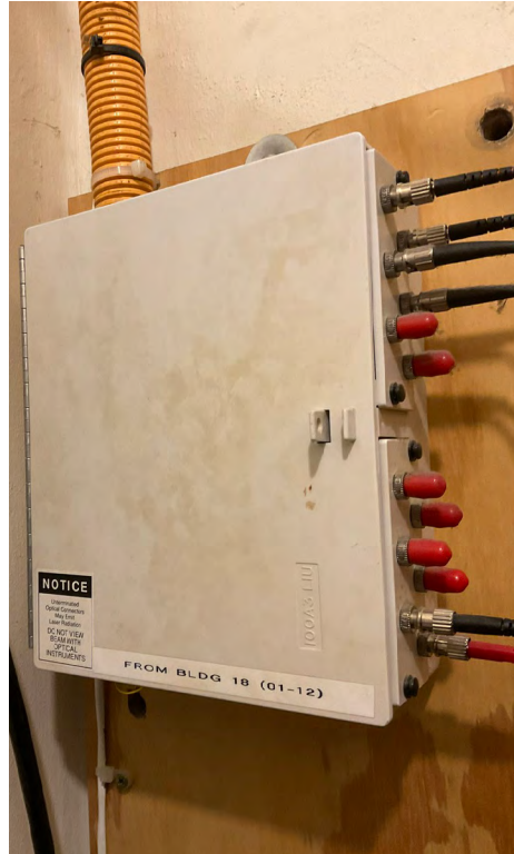
Existing Fiber Cabinet.
