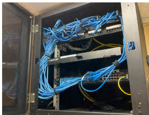
Existing Telecom Enclosure.
