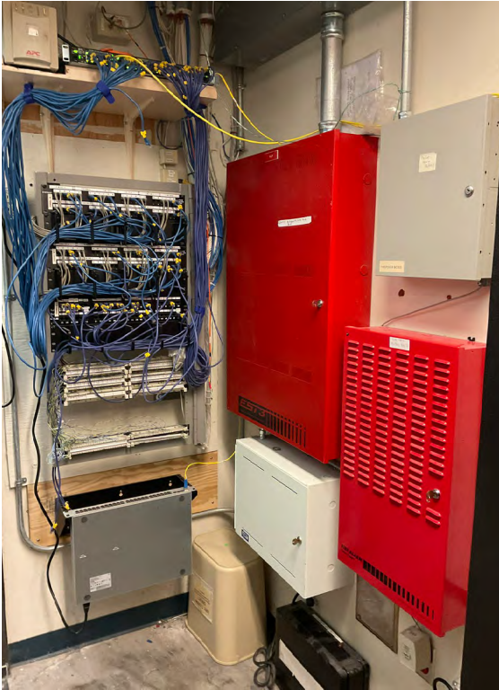
Existing Telecom Room.
