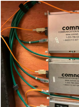
Existing Media Converters.
