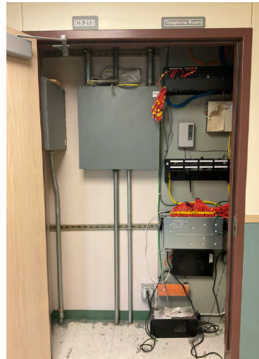
Existing Telecom Room.
