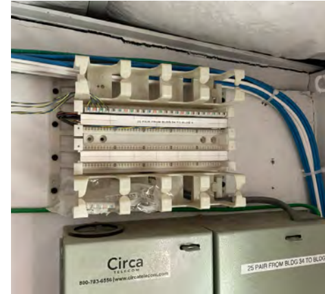
Existing Voice Patching.
