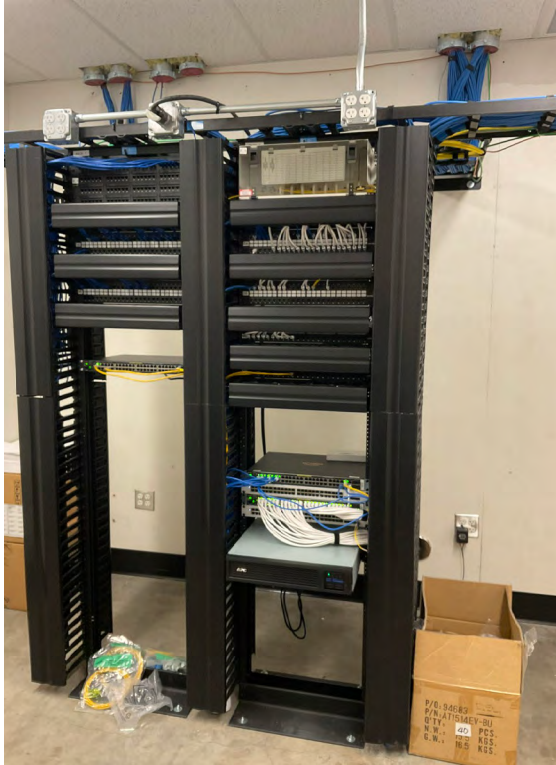
Existing Telecom Racks.
