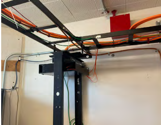
Existing Ladder Tray.
