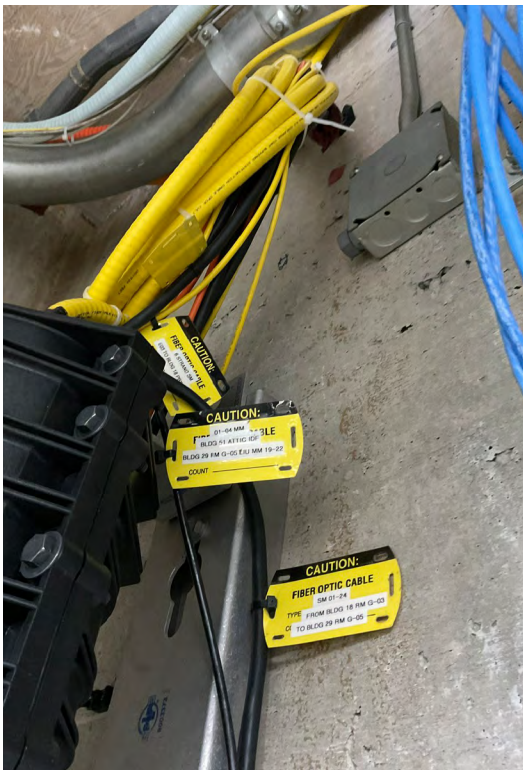
Existing Fiber Cabling.
