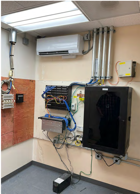
Existing Telecom Equipment.
