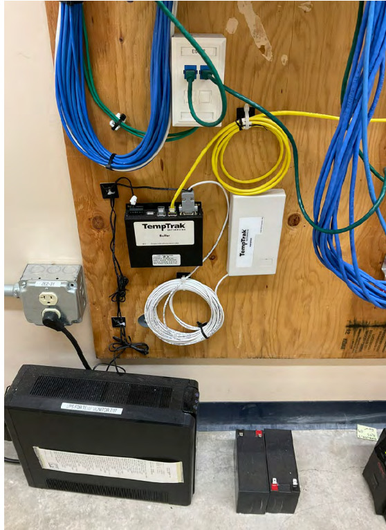
Existing Wall-Mounted Equipment.
