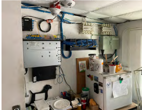
Existing Telecom Room.
