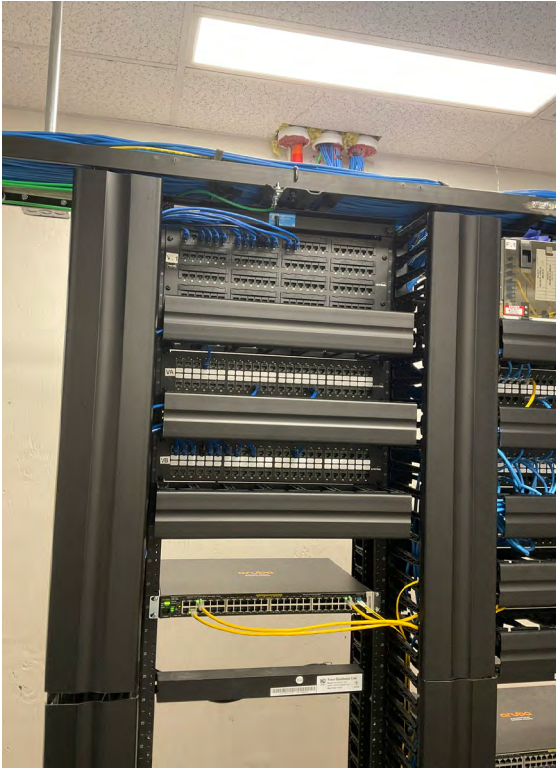
Existing Telecom Rack.
