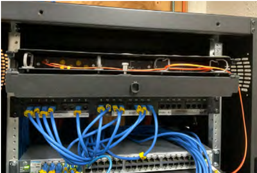
Existing Fiber Patching.
