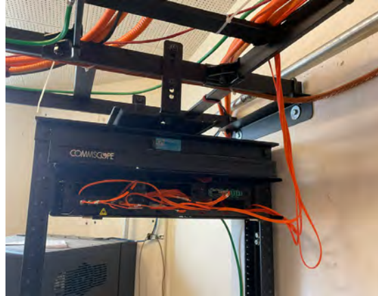
Existing Telecom Rack.
