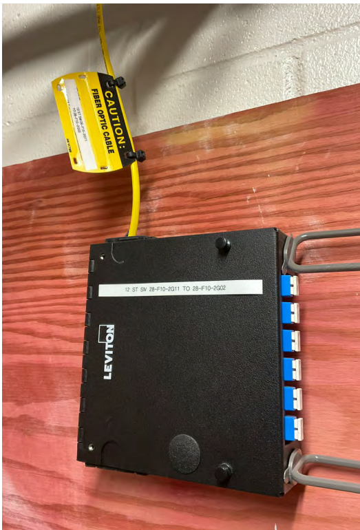
Existing Unused Fiber Cabinet.
