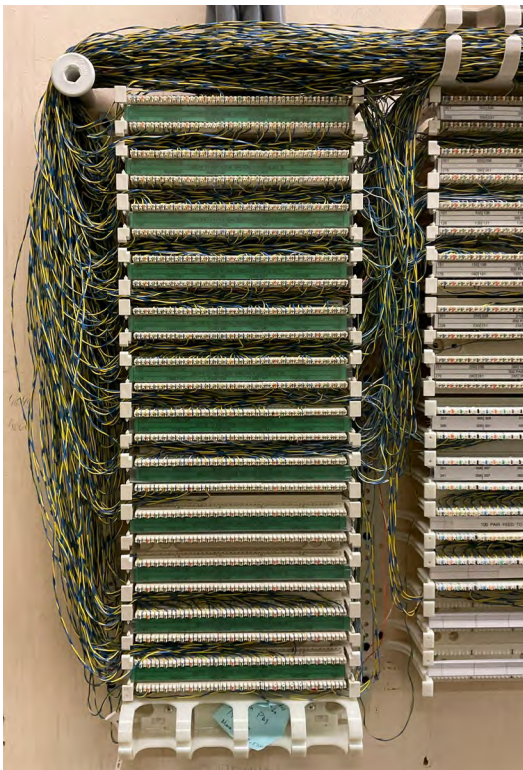
Existing Voice Patching.
