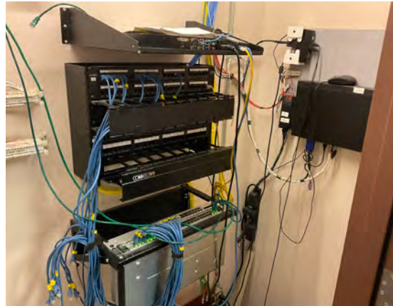
Existing Telecom Rack.
