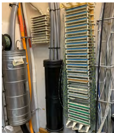
Building 17 Voice Backbone Cabling.
