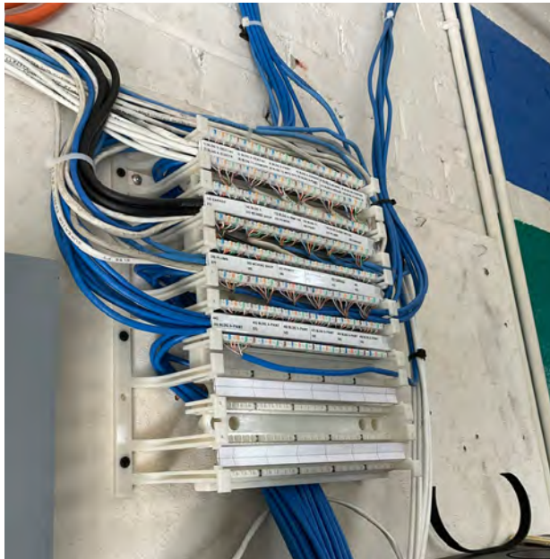
Existing Voice Patching.
