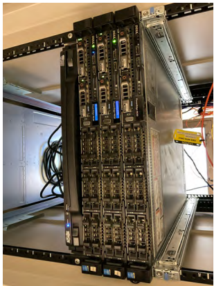
Existing Server Equipment.
