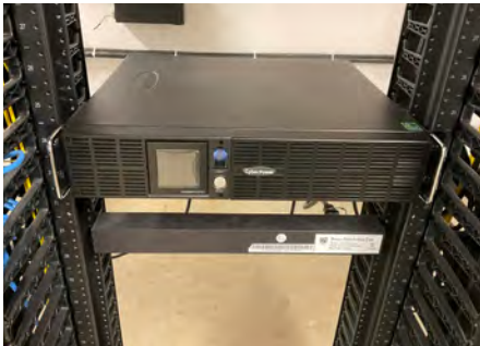
Existing Nonfunctioning UPS.
