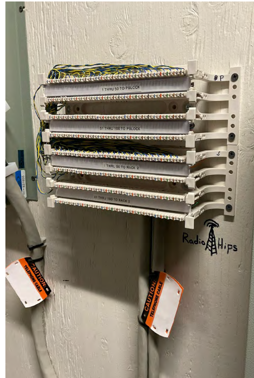
Existing Voice Patching.
