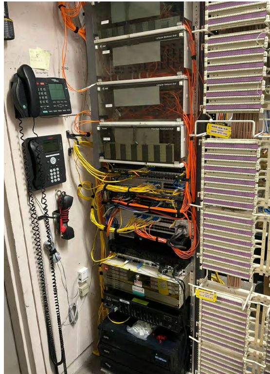
Existing Telecom Racks.
