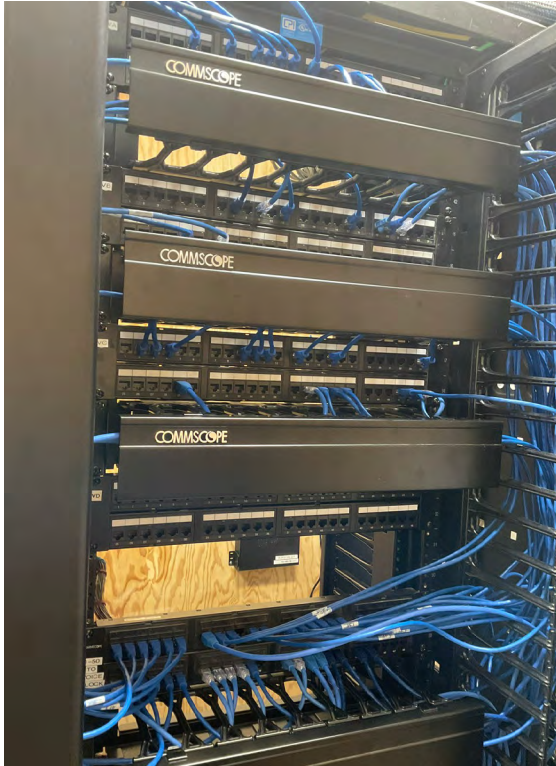
Existing Telecom Rack.
