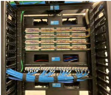
Existing Voice and Data Patching.
