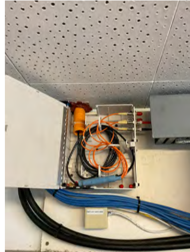
Existing Fiber Cabinet.
