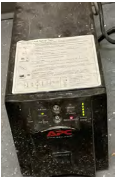
Existing Failing UPS.
