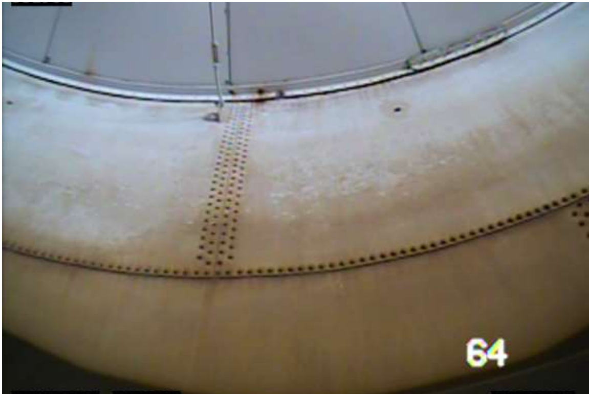
Photo shows the interior roof-to-rim angle connection, which appears to be in good condition.
