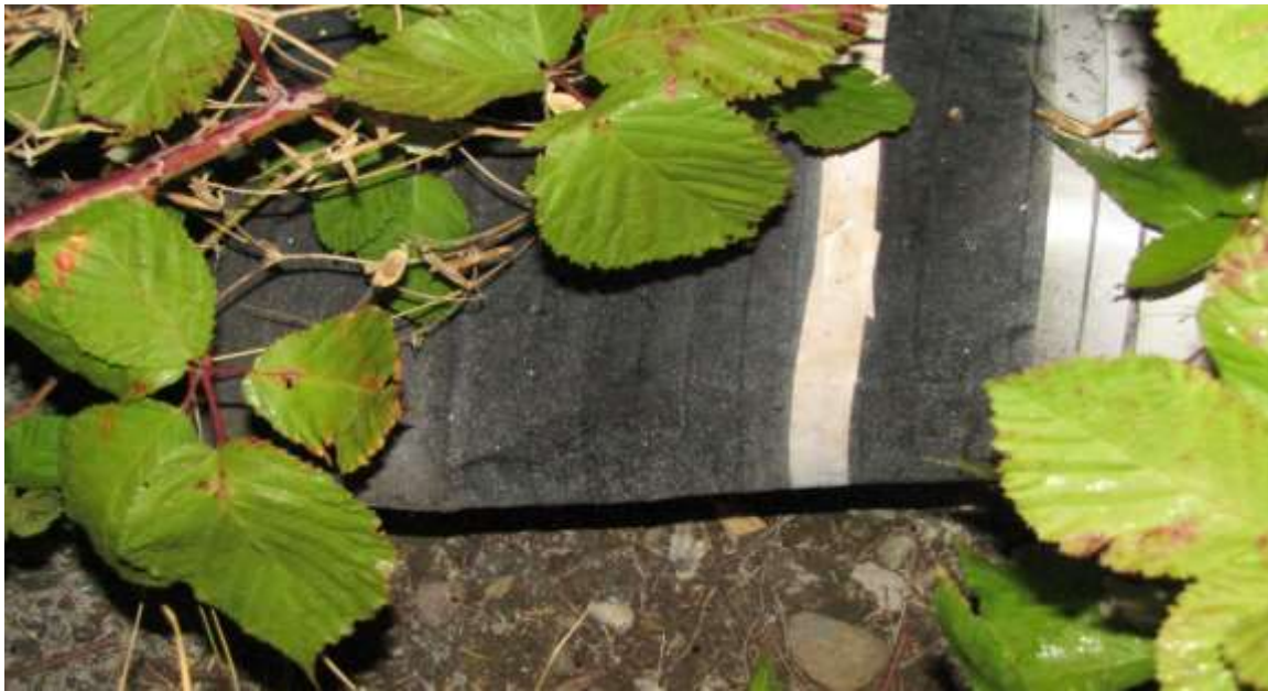
Photos show the 8" overflow pipe system, which is equipped with a flapper valve as required by AWWA D103-09; 7.3: Overflow .
