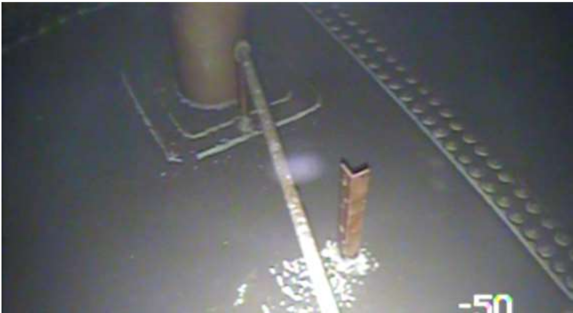
Photos show sediment and debris in the tank interior prior to the performance of the tank clean out.
