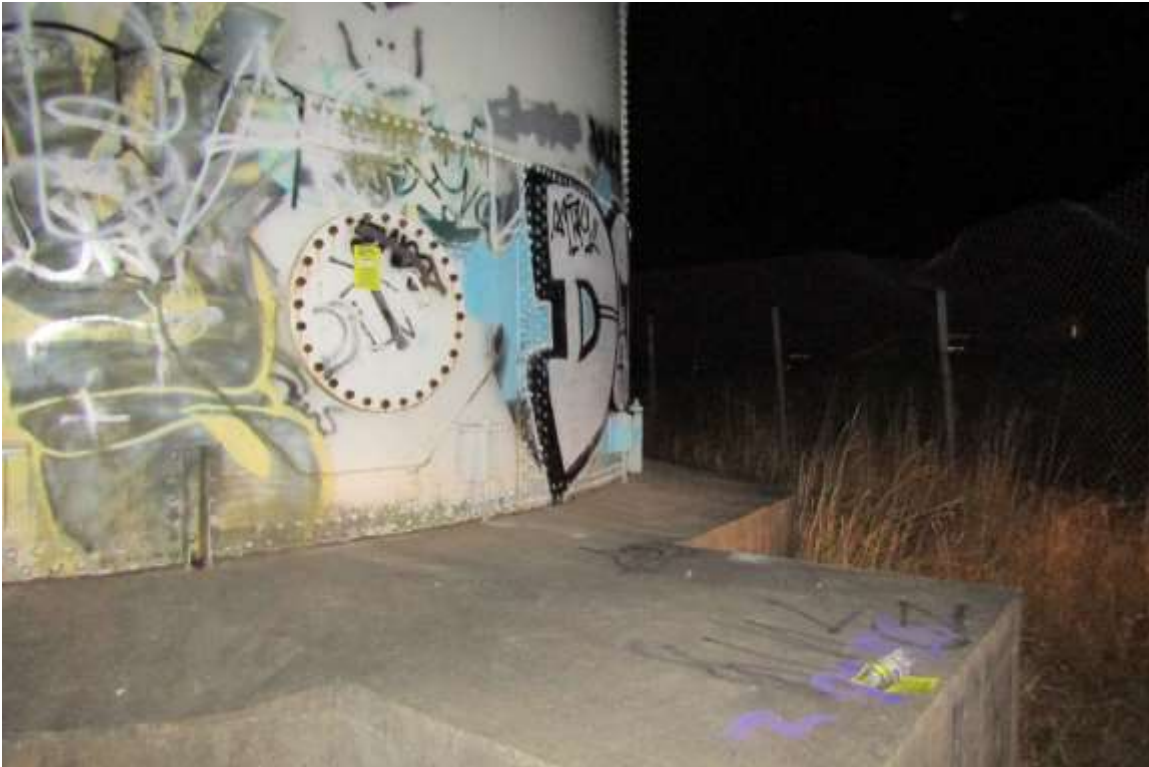
Photo shows the foundation, which is in compliance with AWWA D103-09; 13.5.1: Height above ground and appears to be in good condition.
